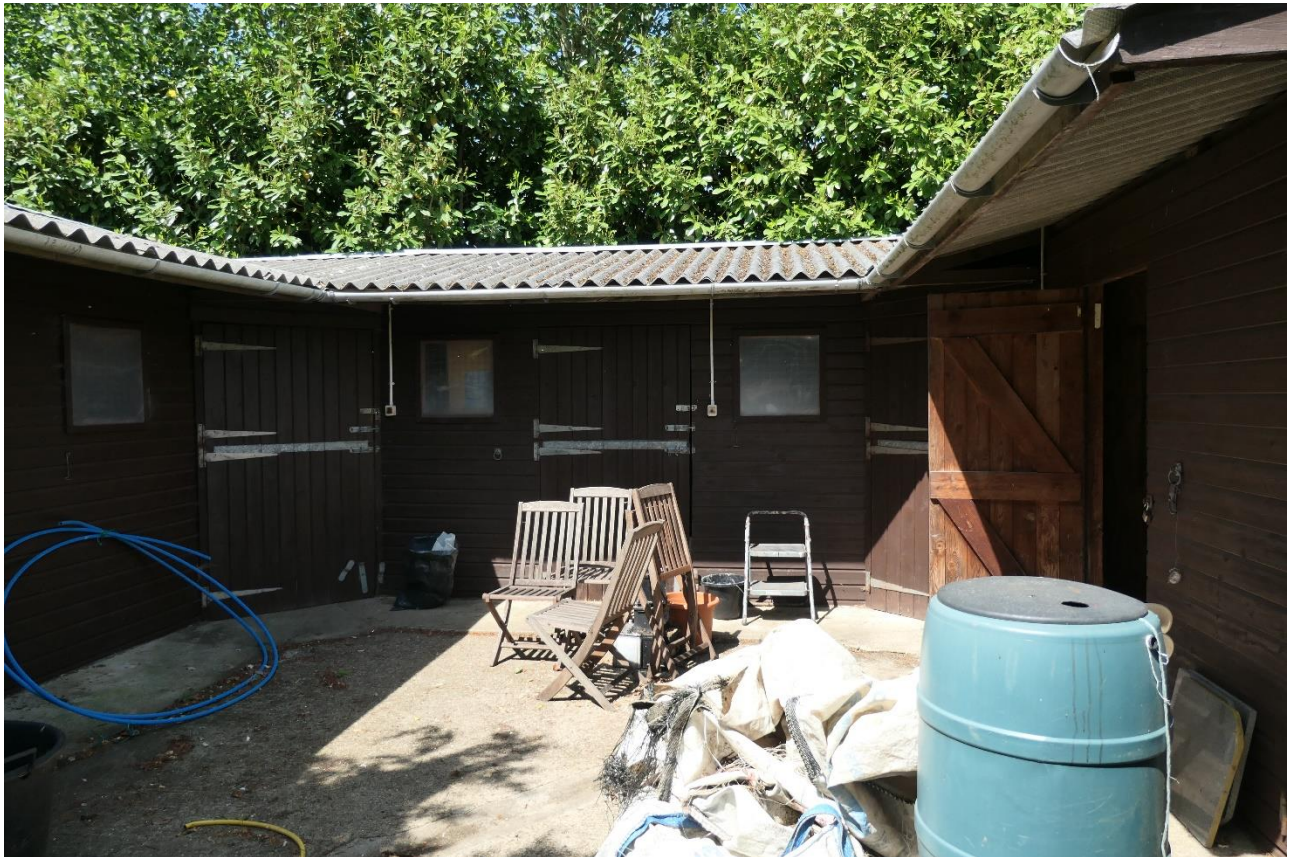
Photo 5: The stables on the application site are rudimentary structures detract from the quality and character of the setting of Hunsdonbury.
