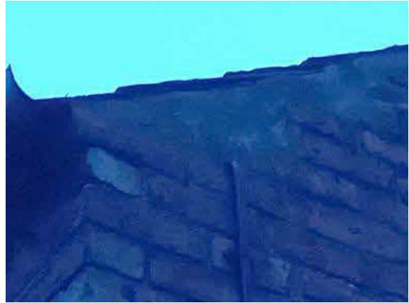
Photograph 2: Gap under tile on eastern elevation with a single bat recorded re-entering building B5
