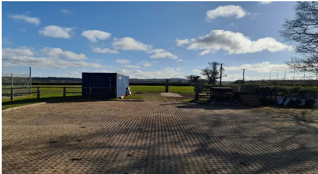
Figure 3: view of the current overspill car park from the current grasscrete car park. (VIVO)
