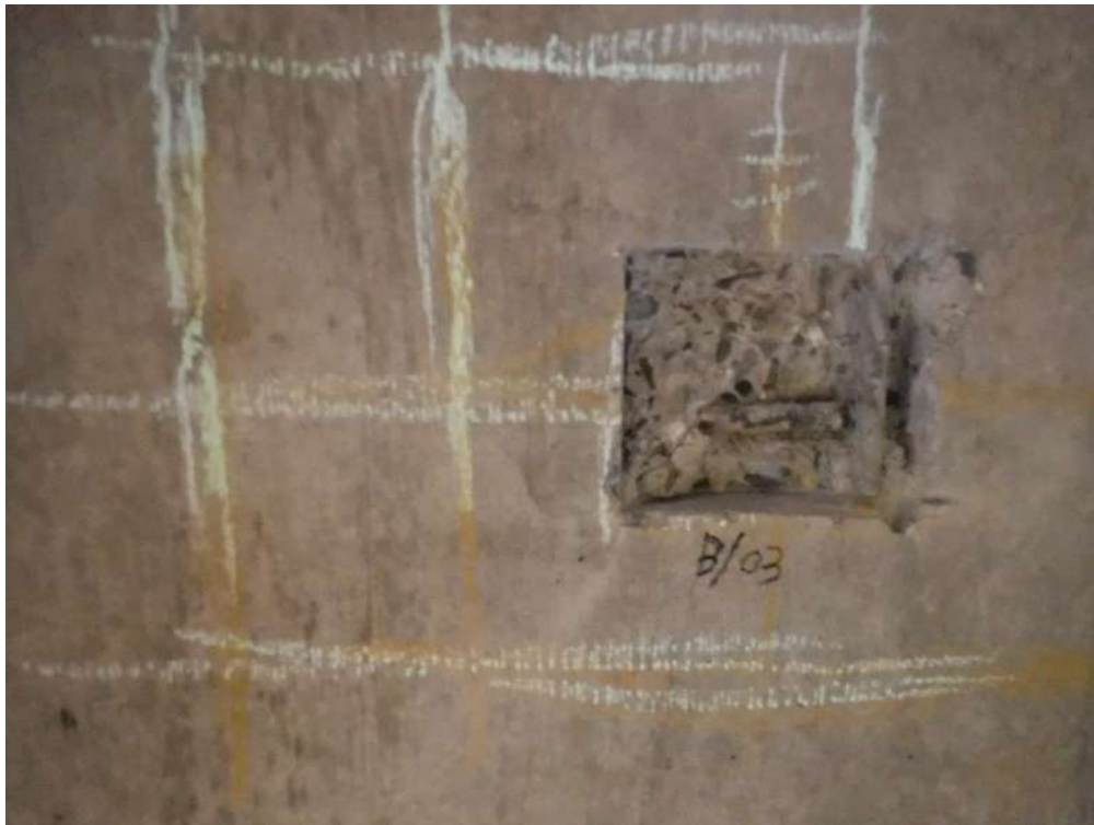
Plate 17 – Showing a general view of breakout B/O3 (underside of 2 nd floor slab).
