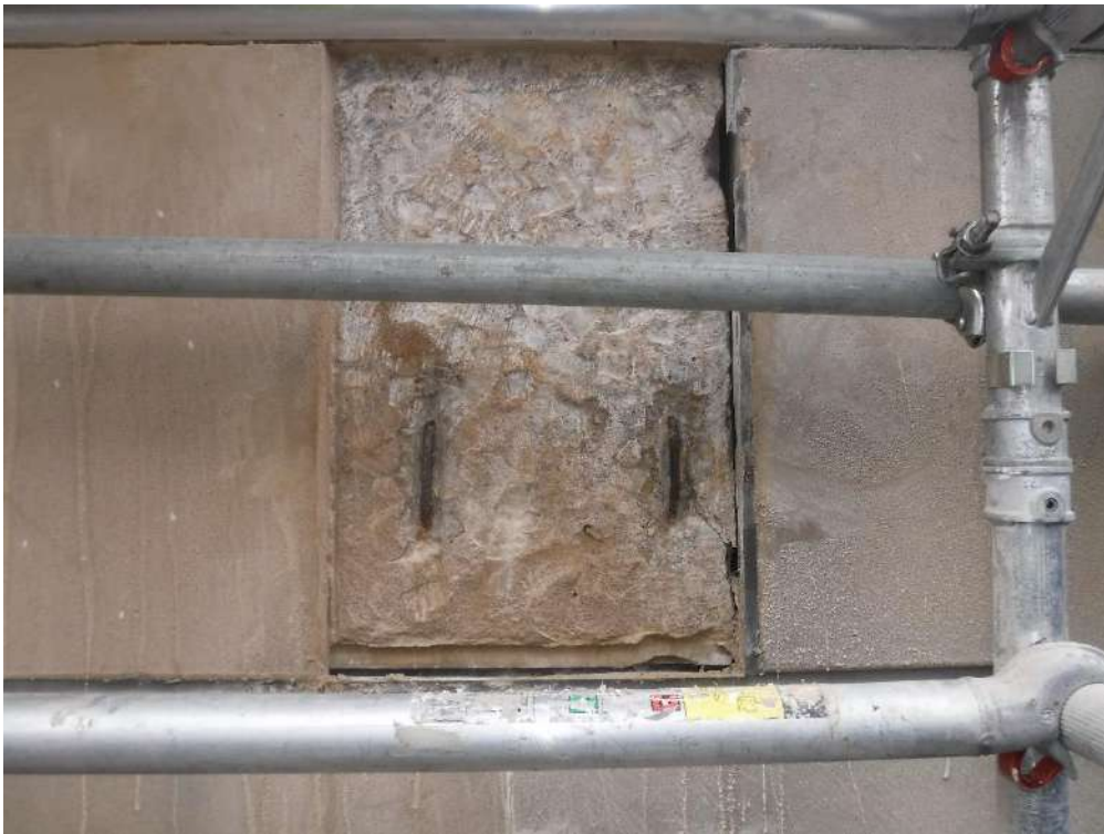
Plate 3 – Showing a general view of Bottom Panel breakout.
