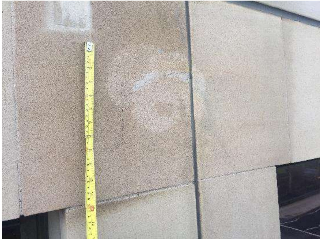
Photograph 3 - Instances of cracking worsening
