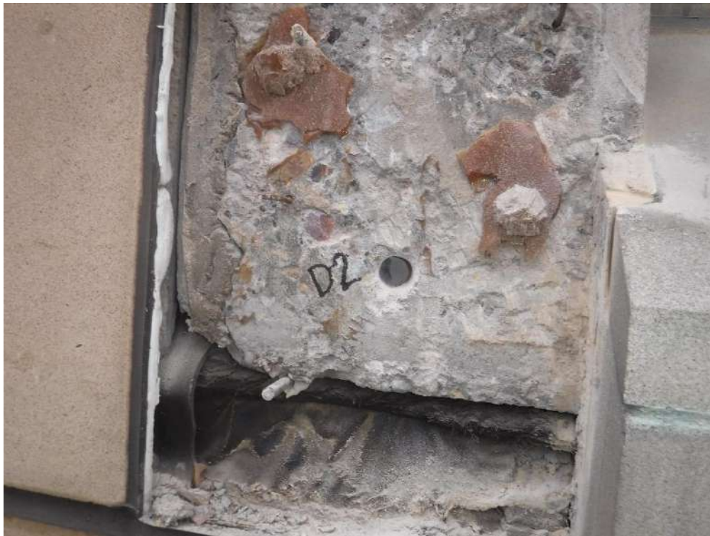
Plate 11 – Showing a close up shot of drill hole D2 on top left-hand side breakout
