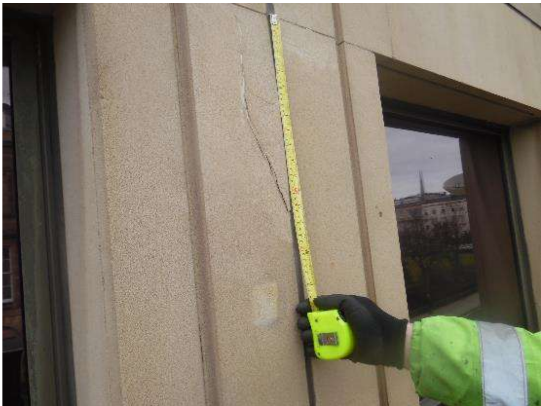
Photograph 4 Example of crack worsening
