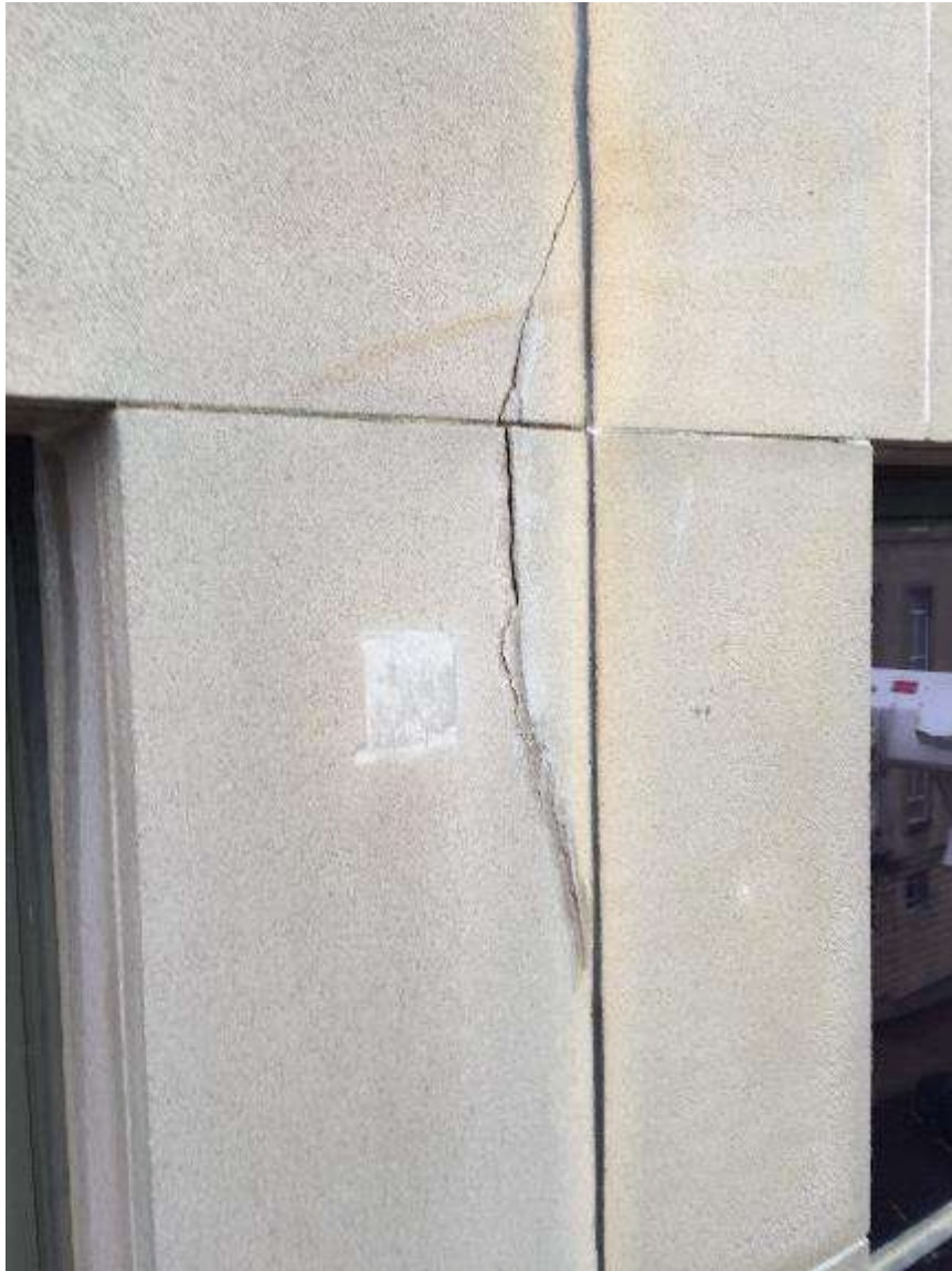
Photograph 5 New Cracking, Blytheswood elevation panel 5/7
