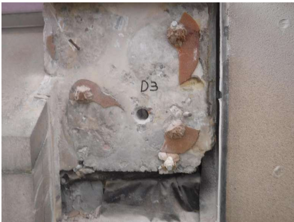
Plate 12 – Showing a close up shot of drill hole D3 on top right-hand side breakout.
