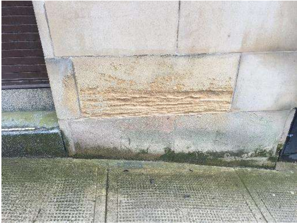
Photograph 8 - General Weathering - Ground level facing
