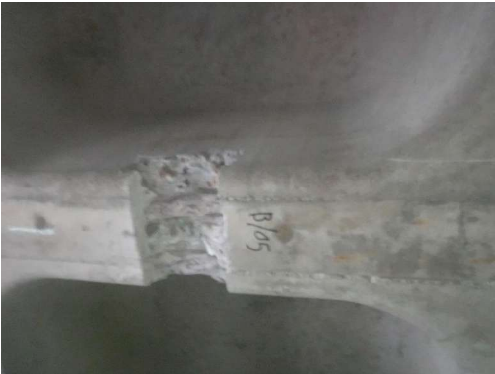
Plate 19 – Showing a general view of breakout B/O5 (underside of 2 nd floor waffle slab rib).
