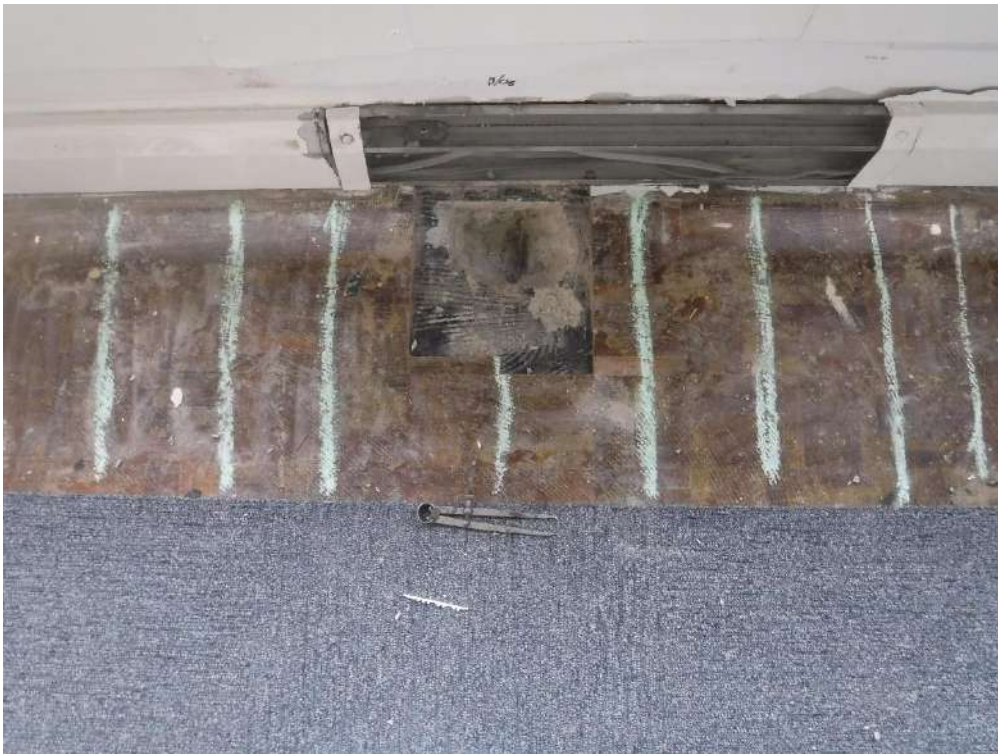
Plate 21 – Showing a general view of breakout B/O6 (top of 3 rd floor slab).
