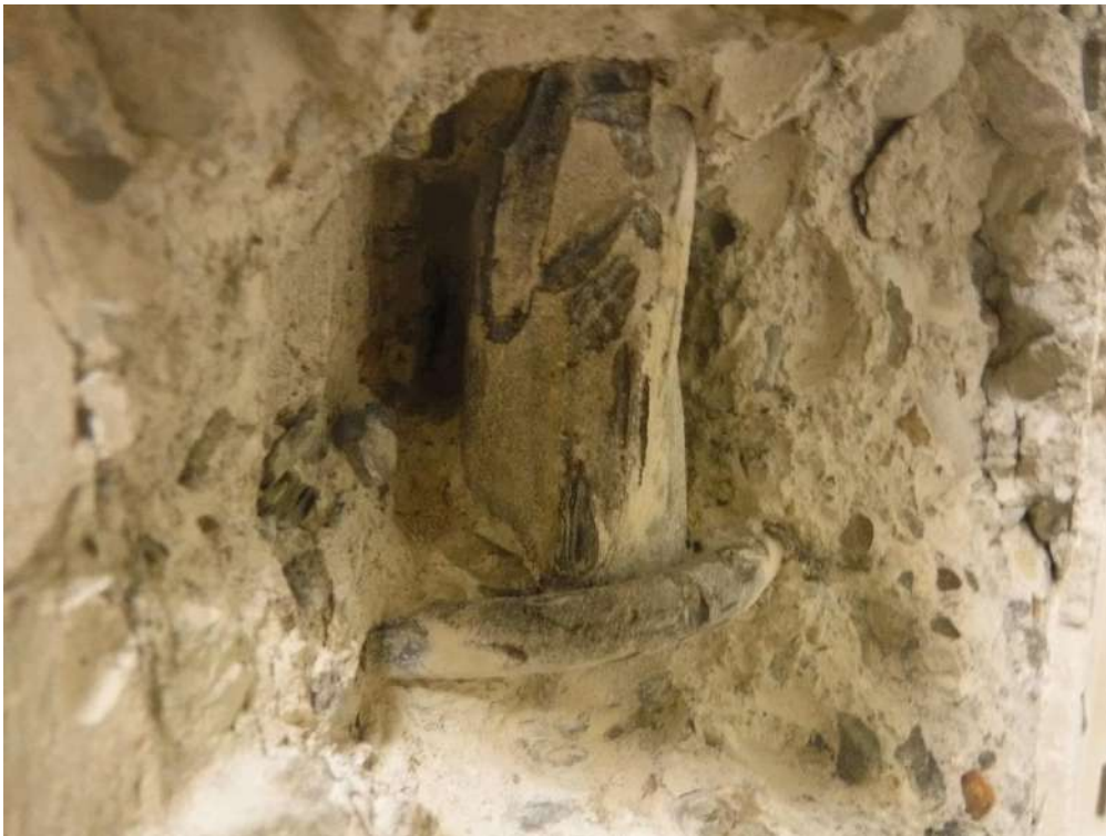
Plate 25 – Showing a close up view of breakout B/O7. Note link.
