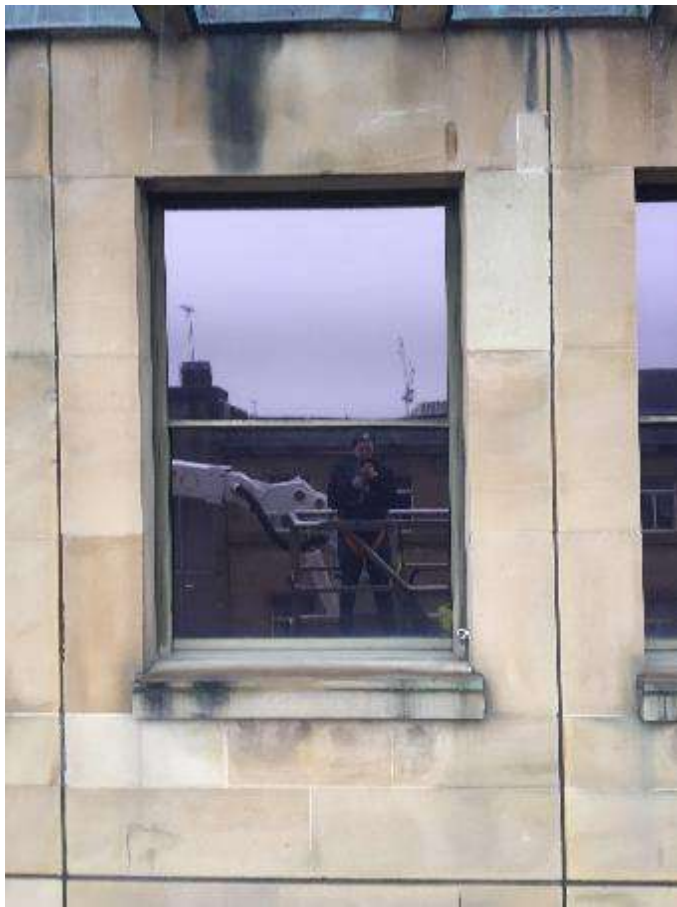
Photograph 7 - General Weathering Pattern
