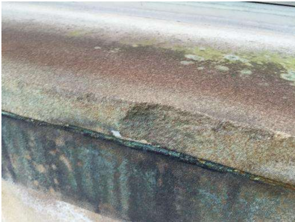
Photograph 9 Cill Weathering and spalling
