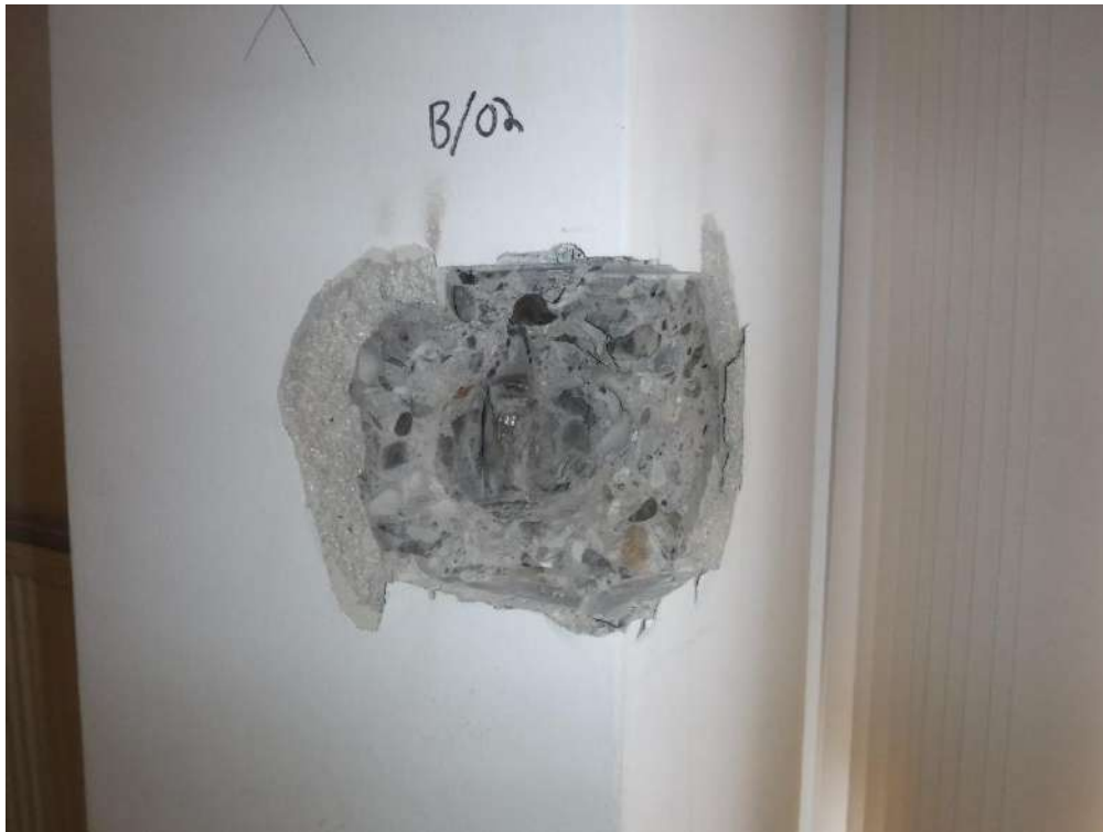
Plate 15 – Showing a general view of breakout B/O2 (perimeter column 1 st floor).
