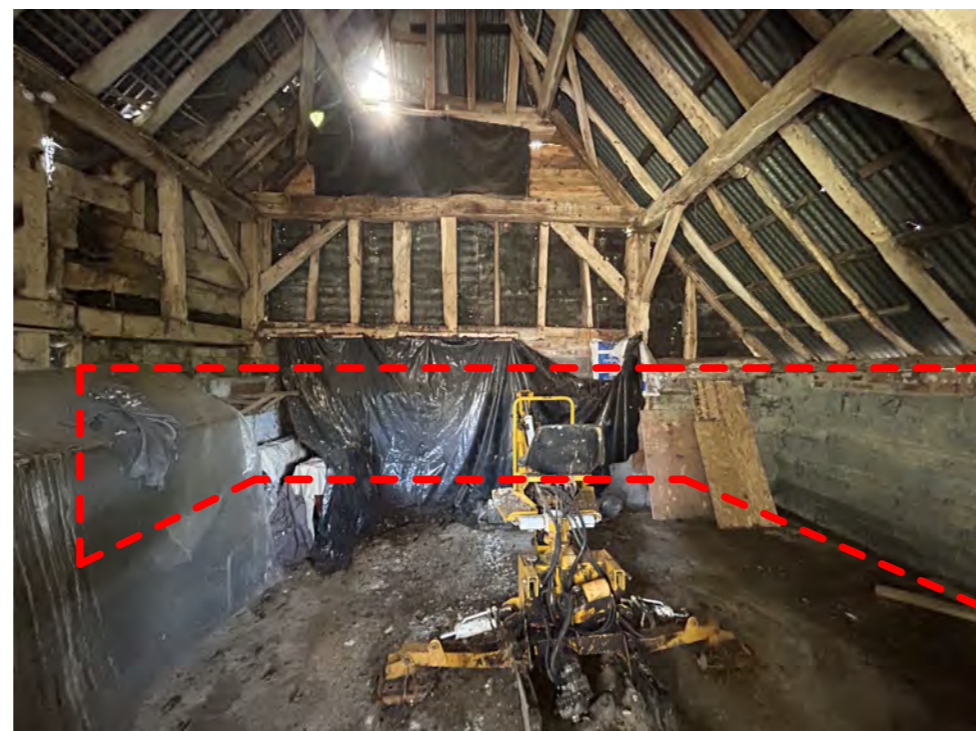
Remove block walls, new glass screen, restore timber framing where possible & around new openings
