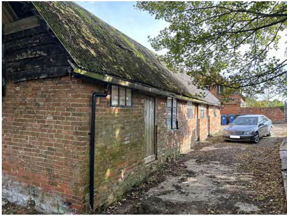
Elevation to garden, windows to be boarded to new upper floor, doors to have low level glazing for new lower level
