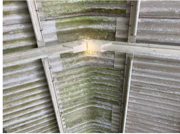
Photo 8: Ridge of Building 2, with no ridge beam present and small gaps at the apex joins filled with dirt and debris
