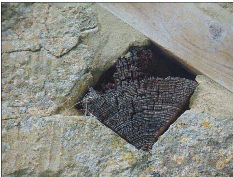
Above: the partially rotted end of a roof timber in the cottage's southern elevation
