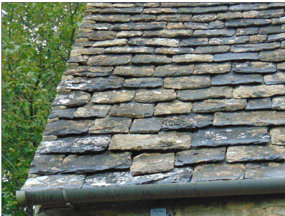
Above: a slipped tile-stone over the western elevation of the cottage
