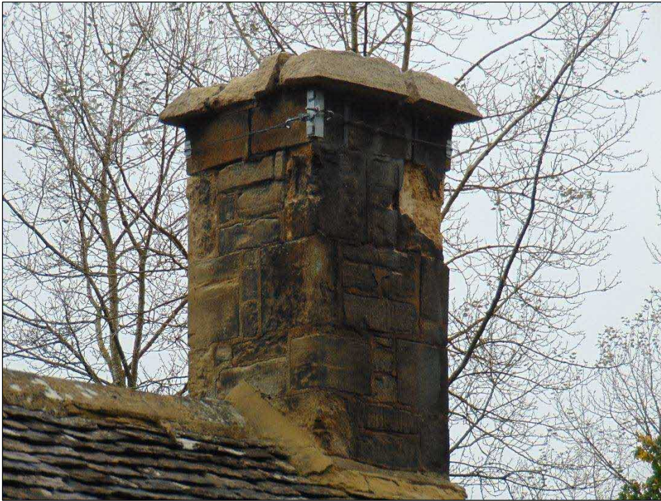
Above: the chimney on the northern elevation of the cottage: in poor condition and with Low bat roost potential
