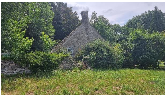
Side gable and fallen walls
