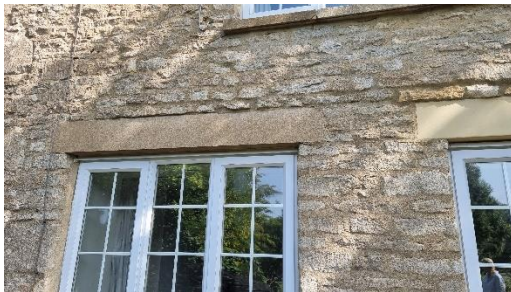
Replaced stone lintels of poor quality
