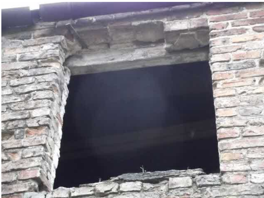
Plate 6. Example of the damaged brickwork at the top of the window opening in the northeast elevation.
