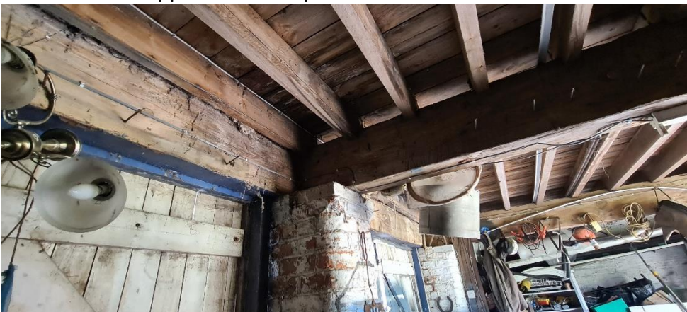
Pic 8 – Timber support and brick pier to the front of the barn
