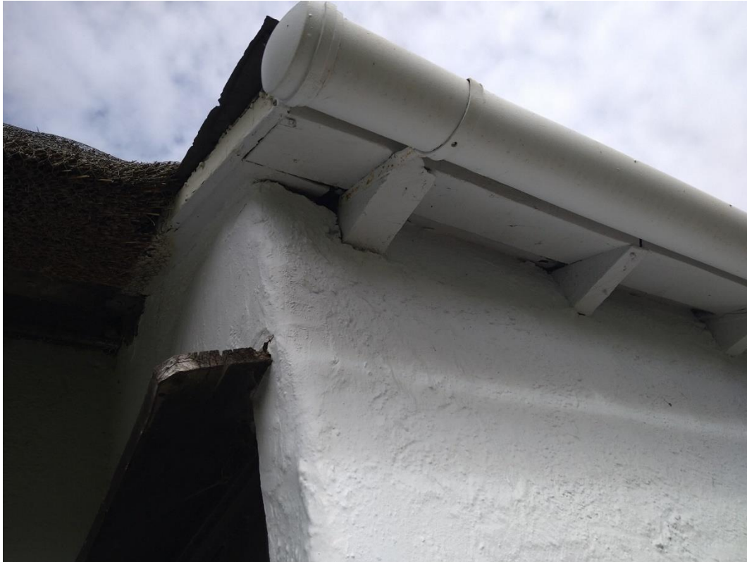
Photo 3: The largest gap under the extension eaves
