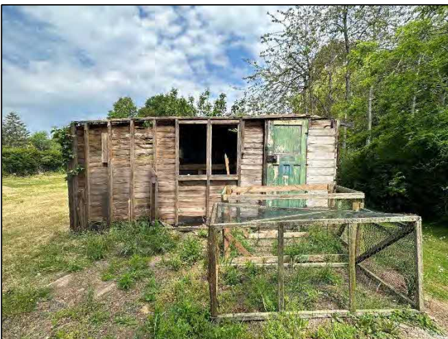
c) Shed close to southern boundary – damaged roof and walls.
