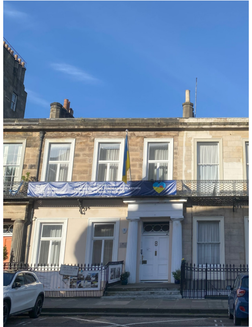
8 Windsor Street – Basement Wall Painted, Partial Upper Wall Painted & Window Reveals Painted
