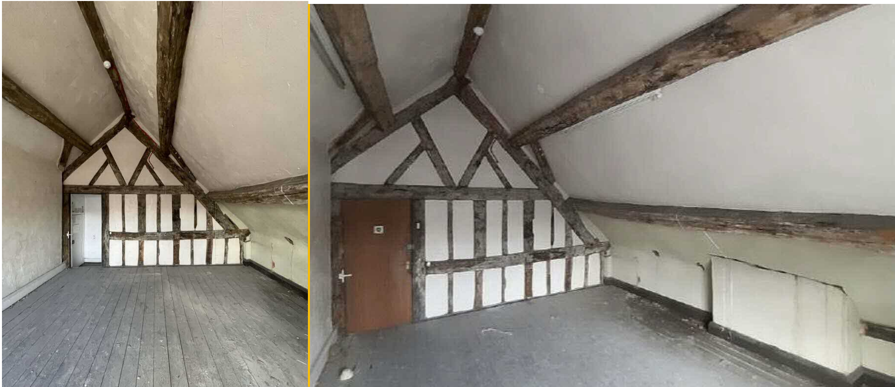
Fig 10. East attic room showing timber frame roofing structure and three oak purlins.
