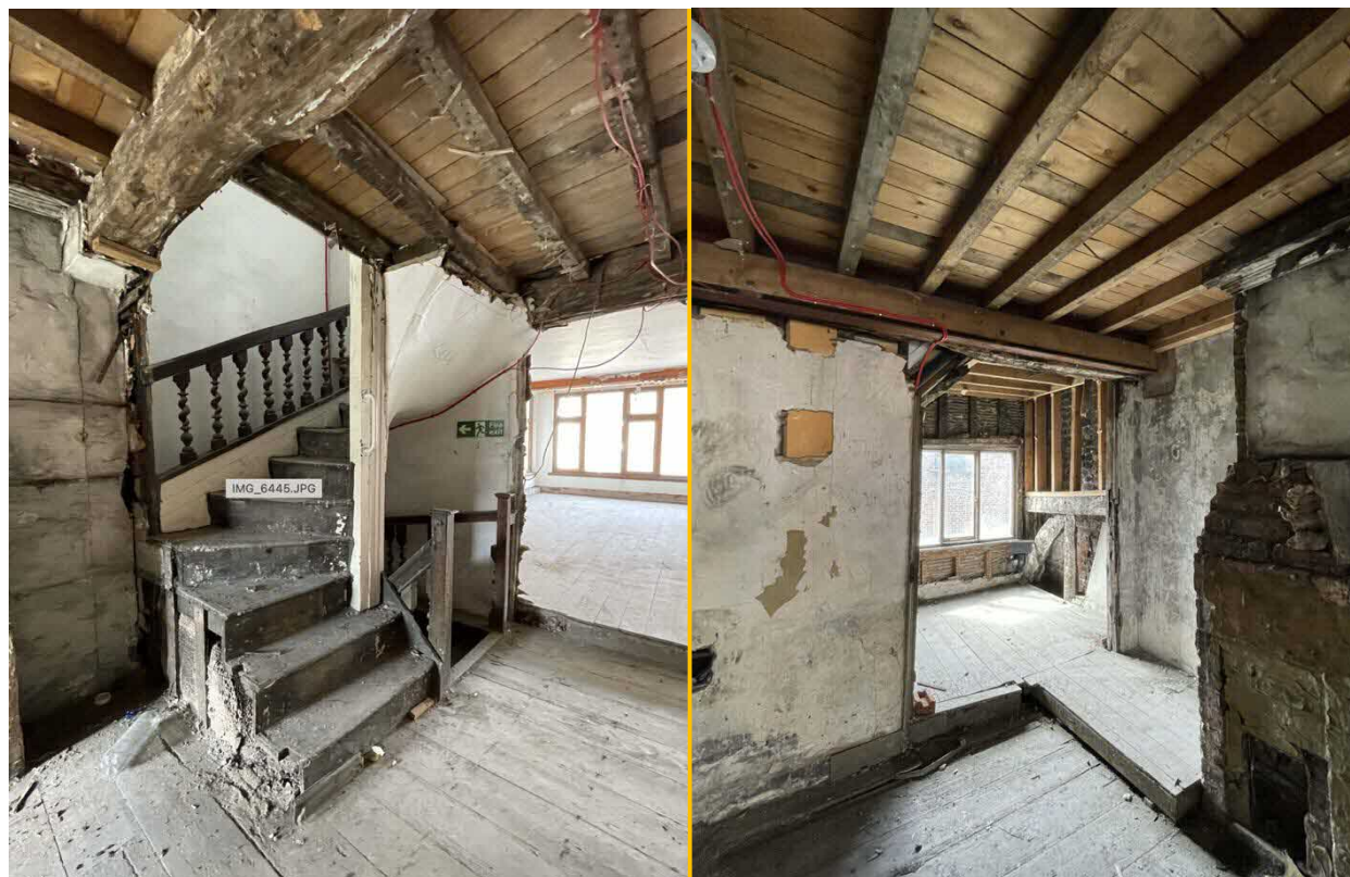
Fig 8. Left: The 17 th century staircase on the Row plus one level; Right The 19 th century fireplace and west facing attic room to rear.
