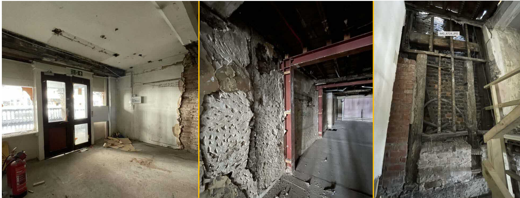
Fig 5. Rows level – left internal view of the Rows doorway; centre: steel goalposts c1973-5; right: timber framing and behind, the south wall of No. 20 Bridge Street
