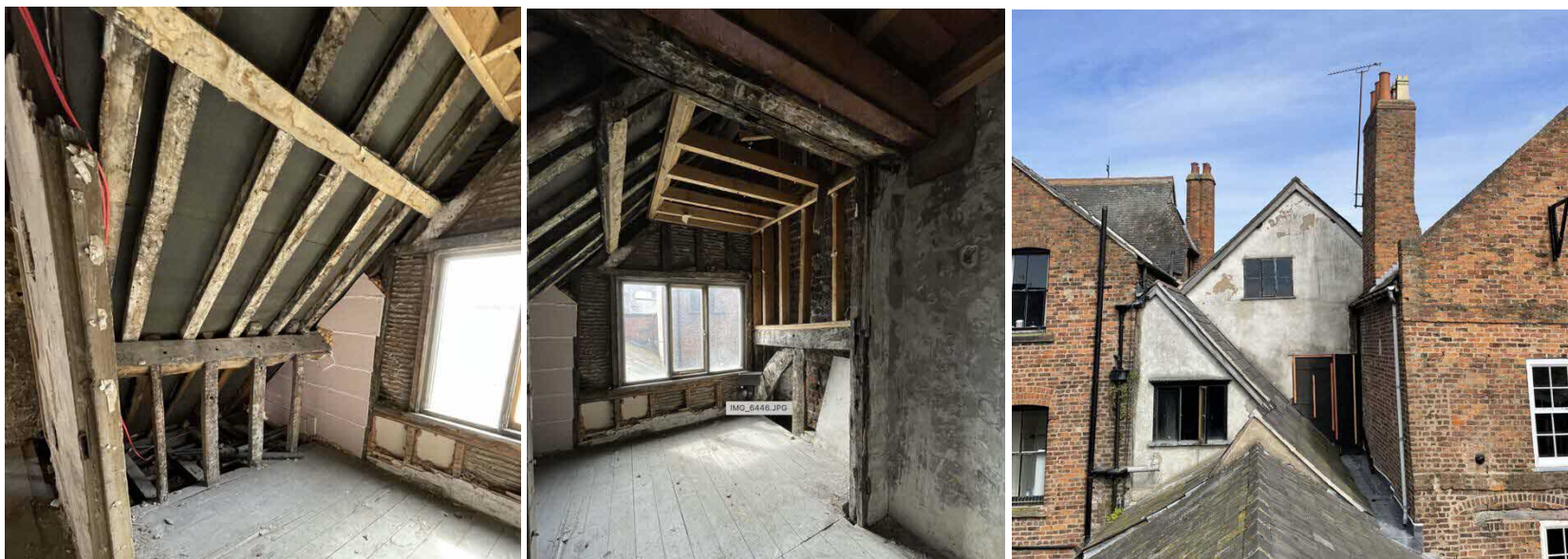
Fig 9. Left: Rear west facing attic room showing 17 th rafters. Middle: note arched braces to rear, and light coloured modern ceiling timbers. It appears that the roof was truncated when No. 20 was built (right), and the timbers of the original roof structure have been pushed back into No. 22 so that they are flat rather than part of the roof structure. Modern windows to rear.
