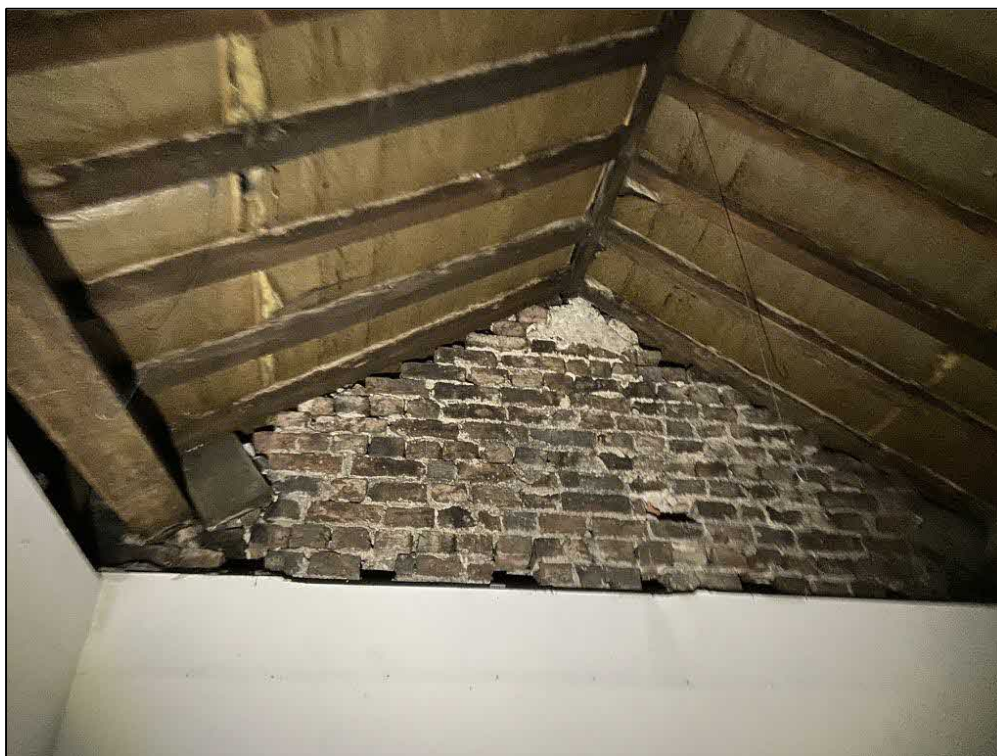
Fig 6: An internal view of the previously pictured section. The internal brick walls are narrow, with no access to any cavities noted.
