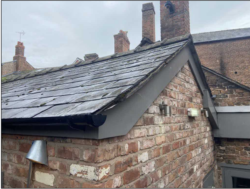
Fig 8: A view of another section to be removed (Building labelled B). This building comprises a single storey, with a standard slate roof. The building is relatively new, and this is reflected by its excellent condition throughout.
