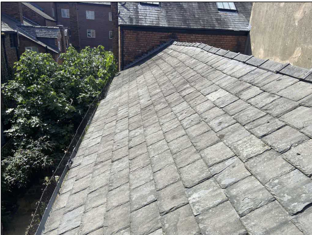
Fig 3: A further view of the roof to be removed as part of the proposals.
