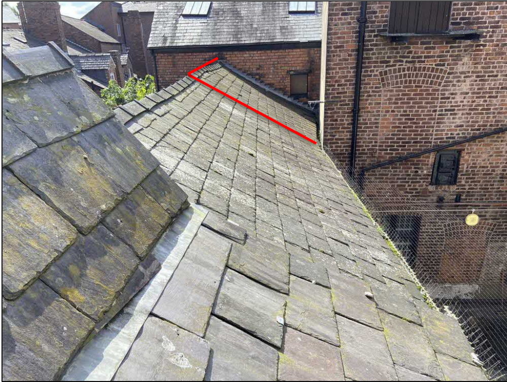
Fig 2: A view of the roof of the section to be removed (labelled building A). The roof tiles and ridge lining was in good condition throughout.
