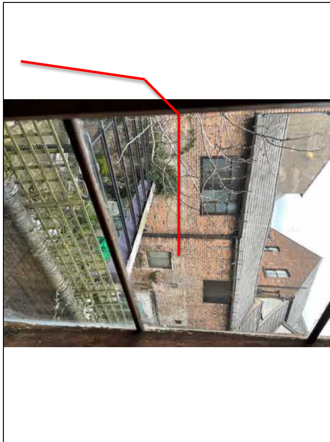
Fig 5: A view from an adjacent retail unit of a subject section for removal. The fascia lining and guttering is in good condition.
