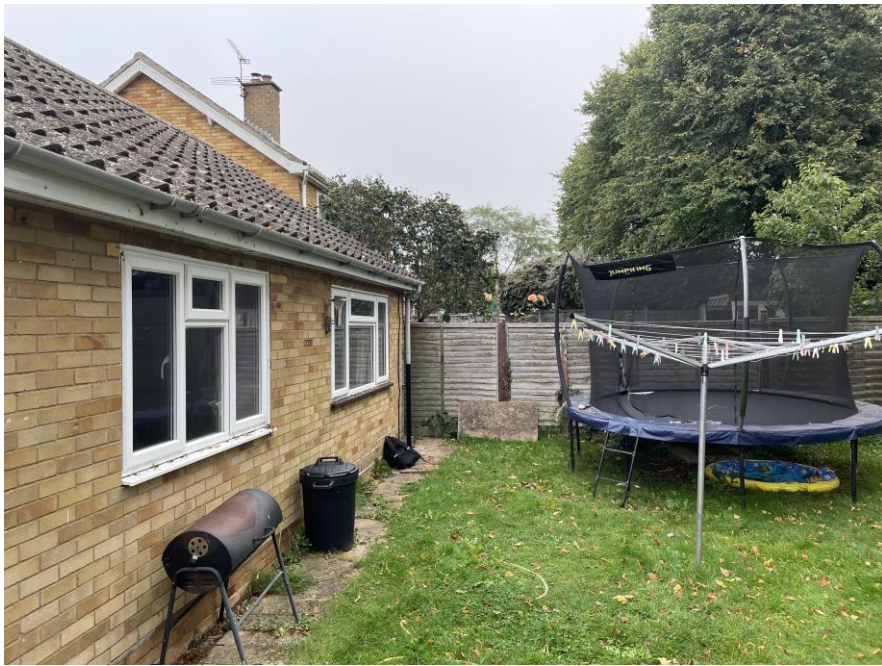
View of the rear of the house with the stepped cracking about the rear left hand corner.
