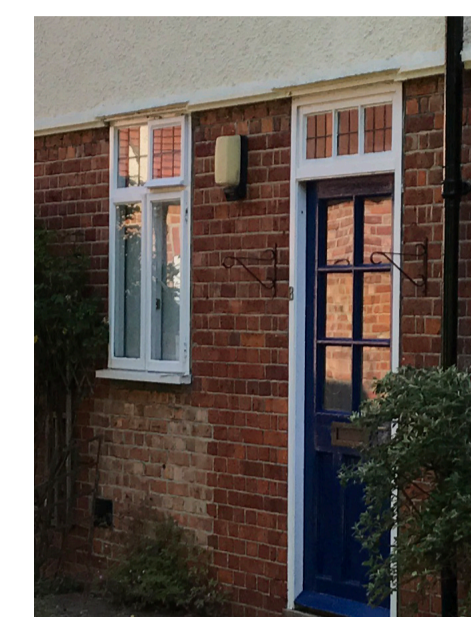
Building mounted light fittings at Lane House
