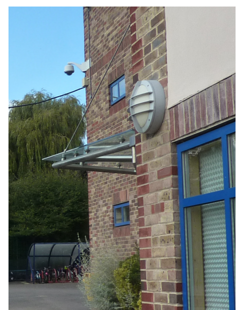
Building mounted light fittings
