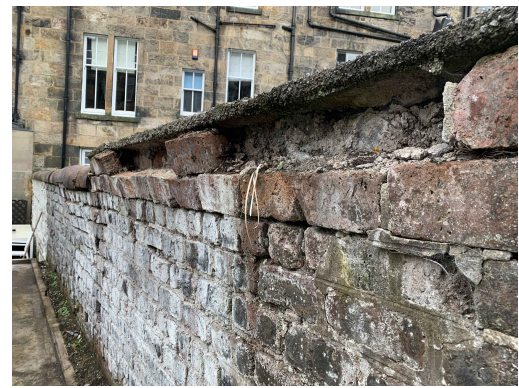
EXISTING DECAYING PARTY WALL
