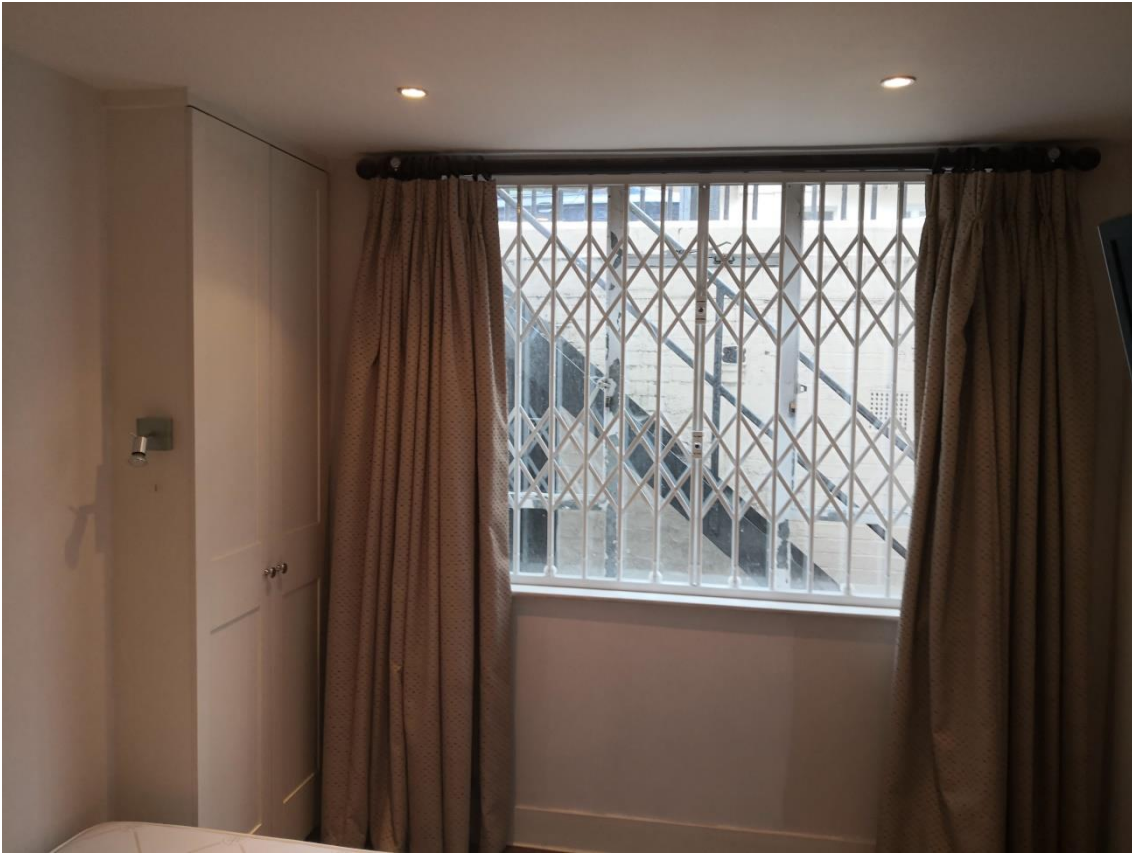
Lower ground floor front room, showing alterations to room and poor condition
