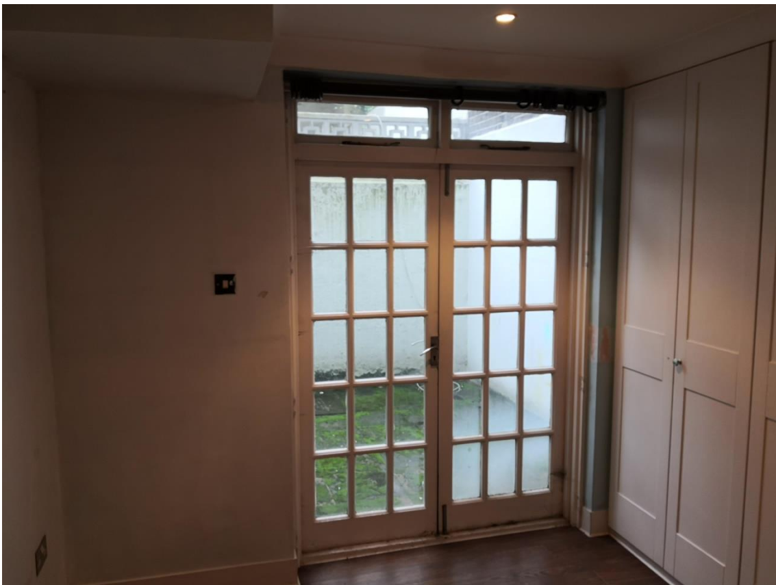
Lower ground floor rear room, similarly showing alterations to room and poor condition
