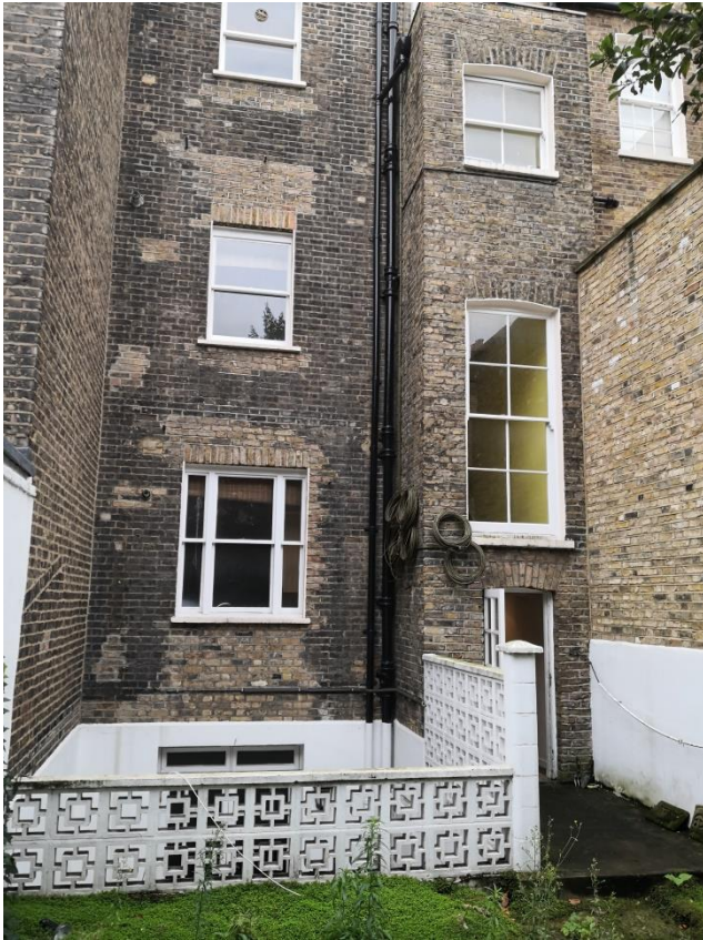
Rear elevation of property, showing alterations to windows and enclosure to basement
