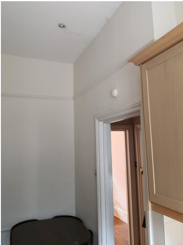
Ground floor rear room, with modifications and partitioning for use as kitchen
