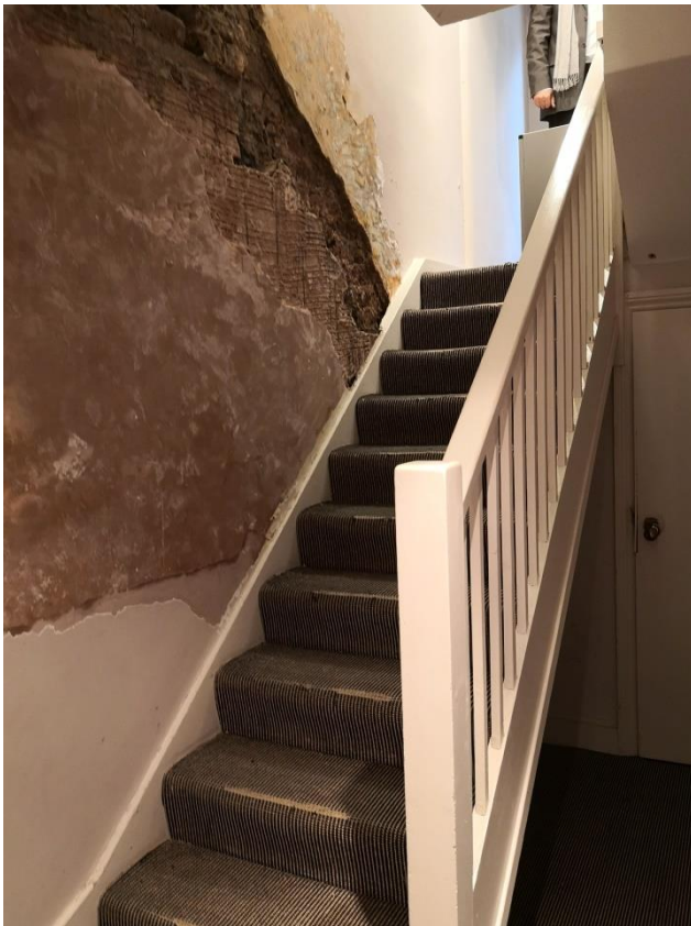
Corridor at lower ground floor, with bathroom to front and modern stairs; line of original stairs still evident from brick scarring
