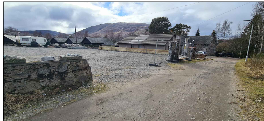
7. View of existing lane and existing stone perimeter wall to be repaired following fire
