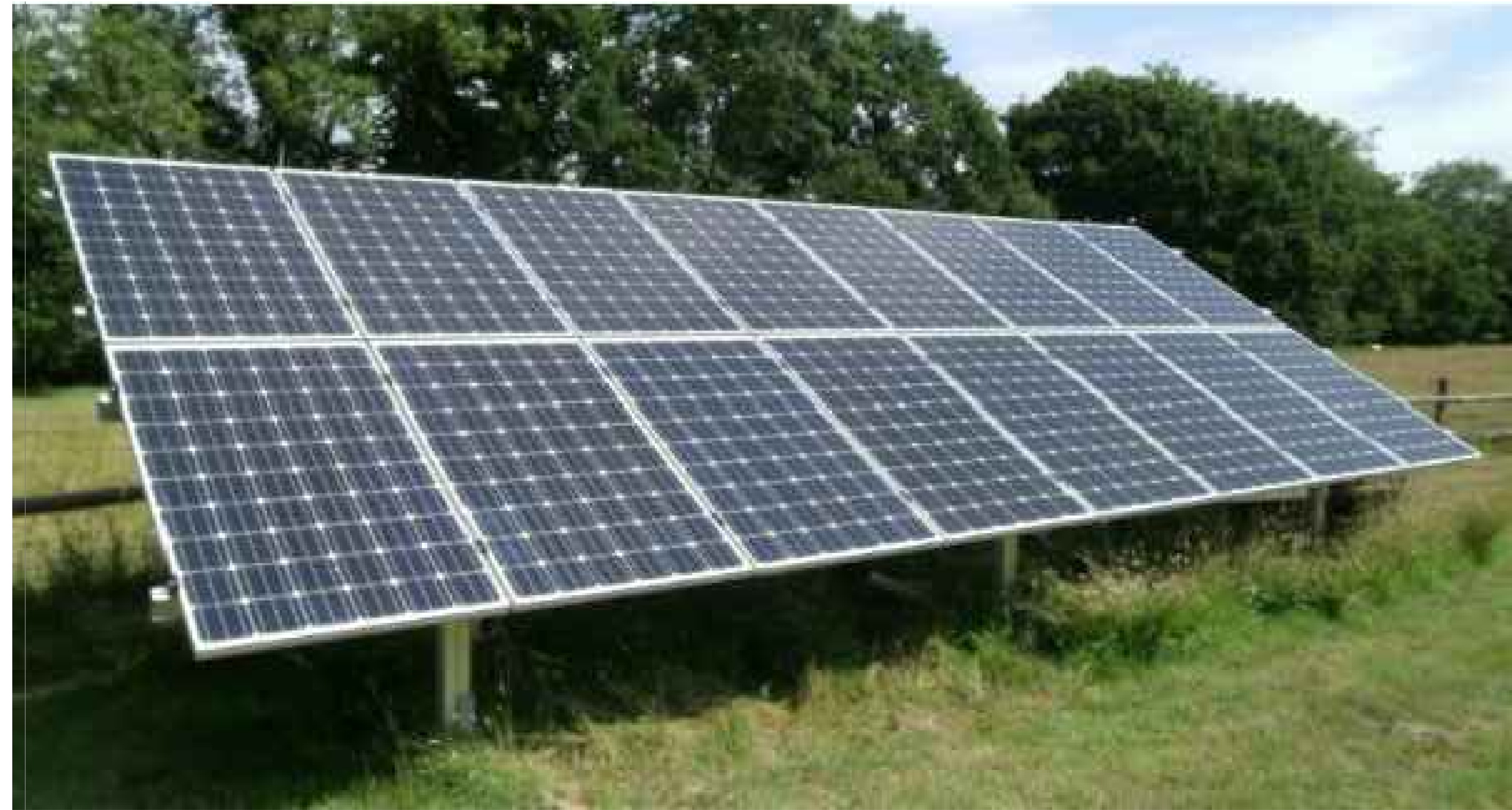
Photo of typical array
