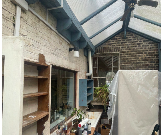
View of the rear wall at ground floor, the original window E.W.02 set within the existing unpainted brick wall
