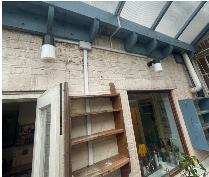
View of side outrigger wall at ground floor, door and window E.D.02 and E.W.03 are relatively new additions
