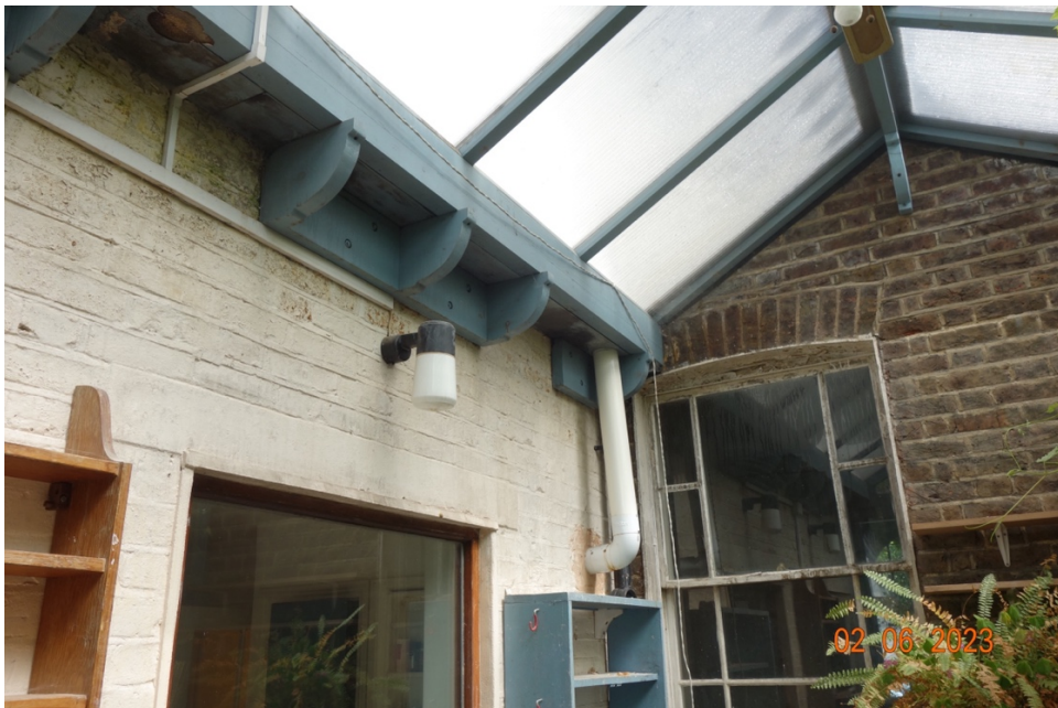
Image 8 Interior of the lamentable existing conservatory showing modern opening in side wall to the rear wing
