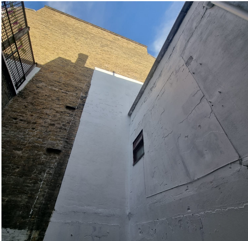
Existing uPVC window @ Rear of 44 Craven Road
