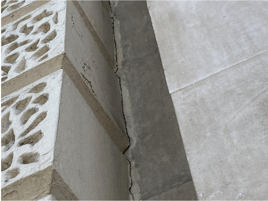
PHOTOGRAPH 11: Crack to joint between 15 Regent Street and adjacent property.
