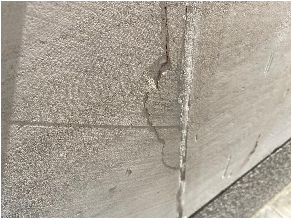
PHOTOGRAPH 8: Spalling stone to the read elevation.
