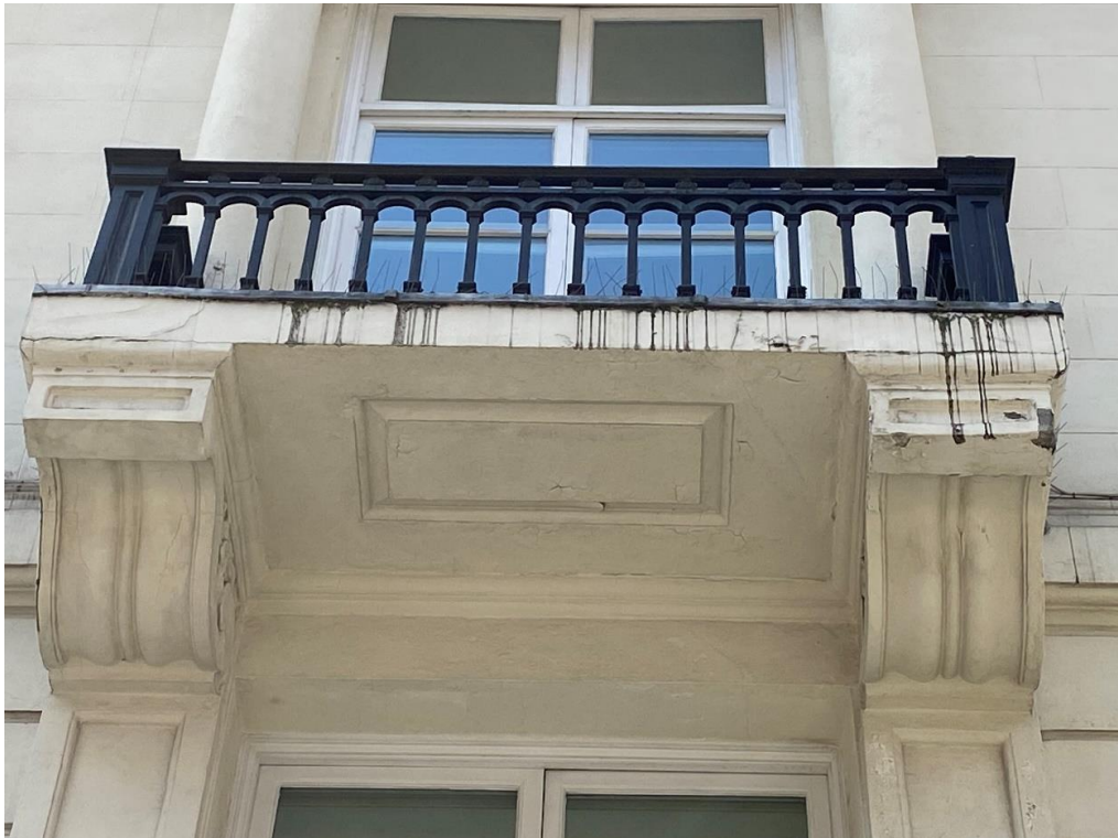
PHOTOGRAPH 10: Splits / cracks to decoration to front elevation. Paint runs visible.
