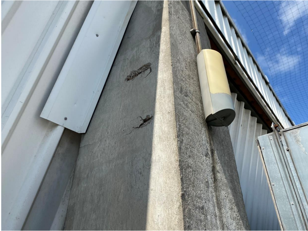
PHOTOGRAPH 5: Spalling to concrete frame.
