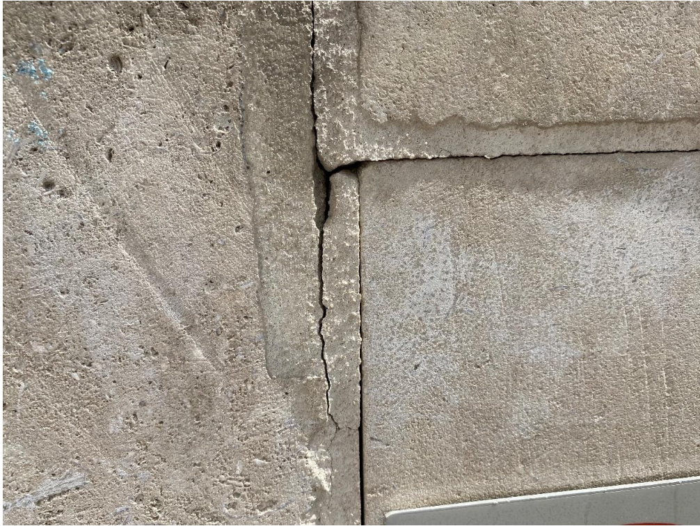
PHOTOGRAPH 9: Loose / Cracked pointing to stone.
