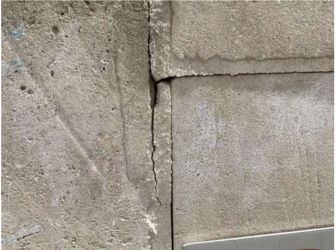
Photo 9: Loose / Cracked pointing to stone.
