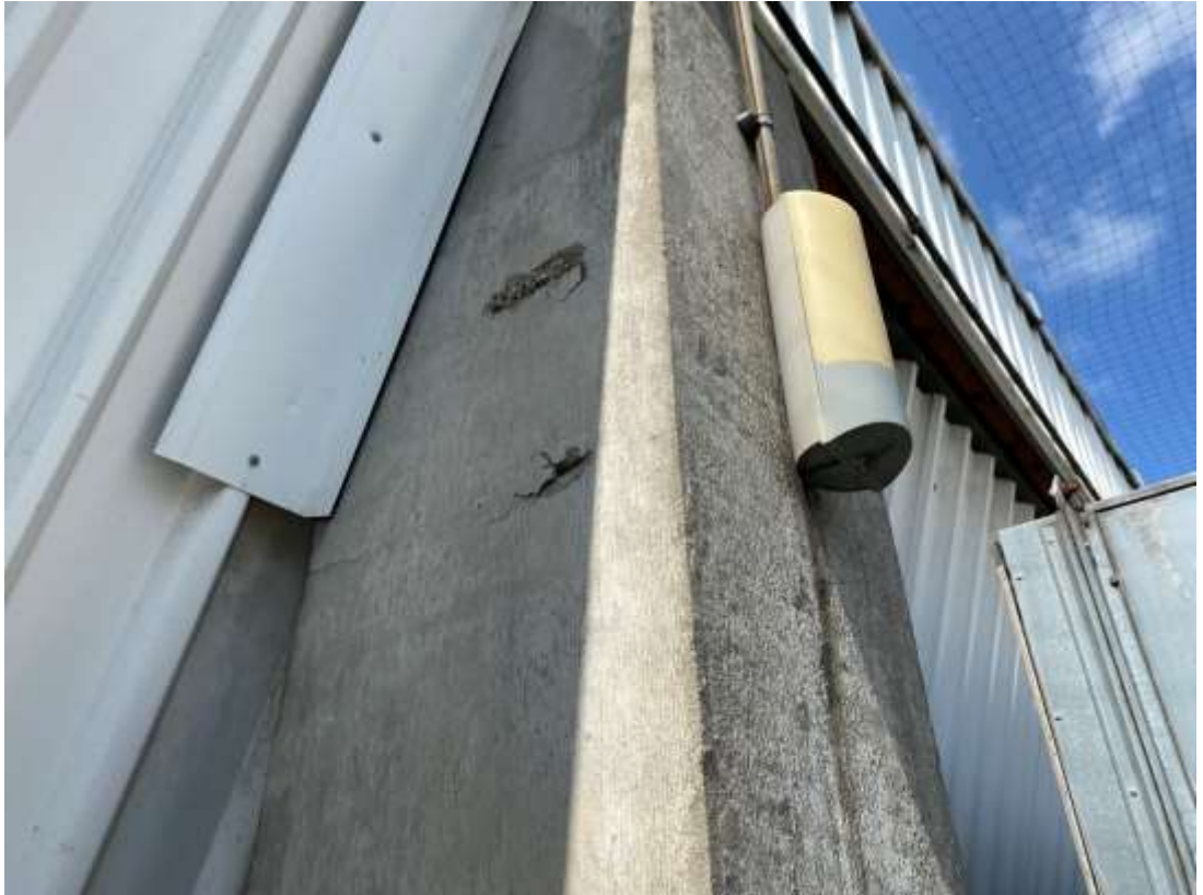
Photo 5: Spalling to concrete frame.
