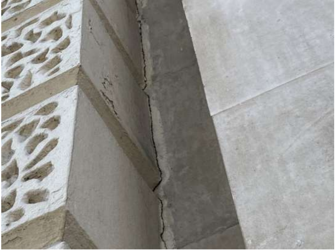
Photo 11: Crack to joint between 15 Regent Street and adjacent property.
