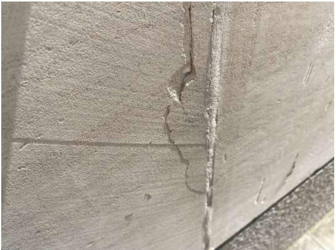
Photo 8: Spalling stone to the read elevation.
