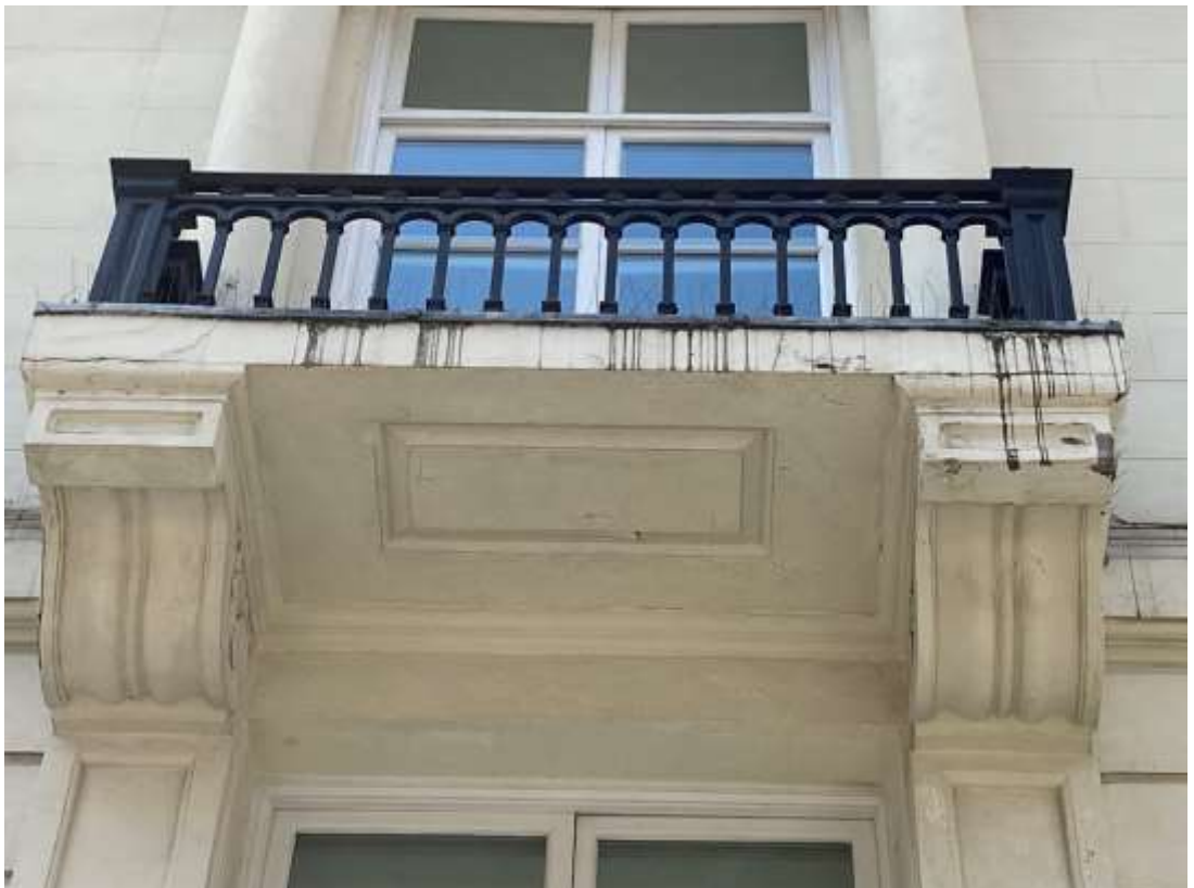
Photo 10: Splits / cracks to decoration to front elevation. Paint runs visible.
