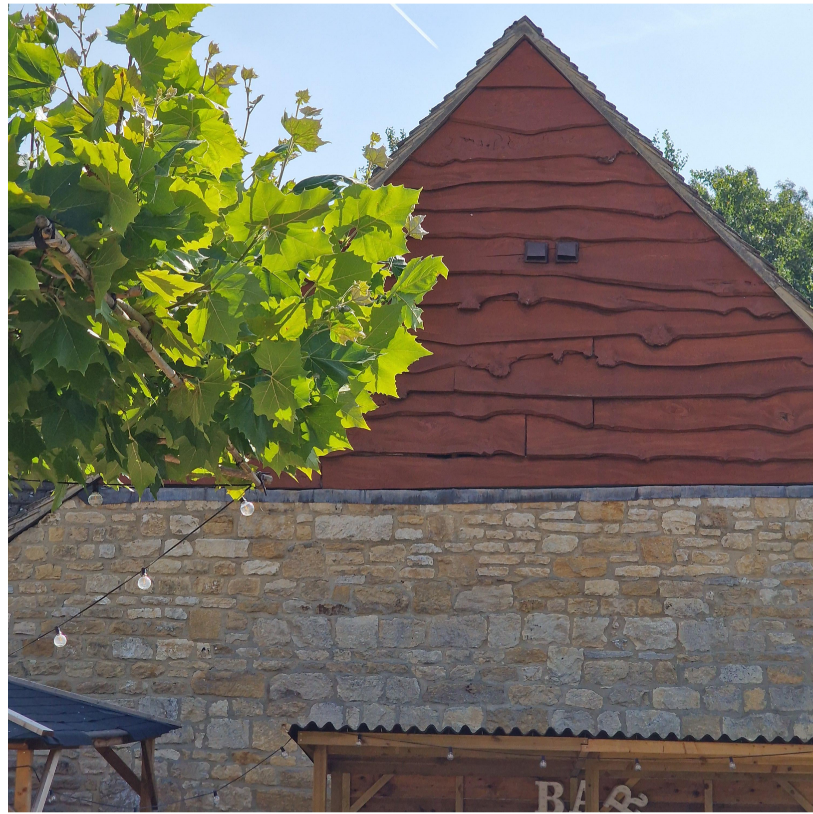
Example of waney edge boarding in Weston Subedge, within the Cotswold District Council conservation area
