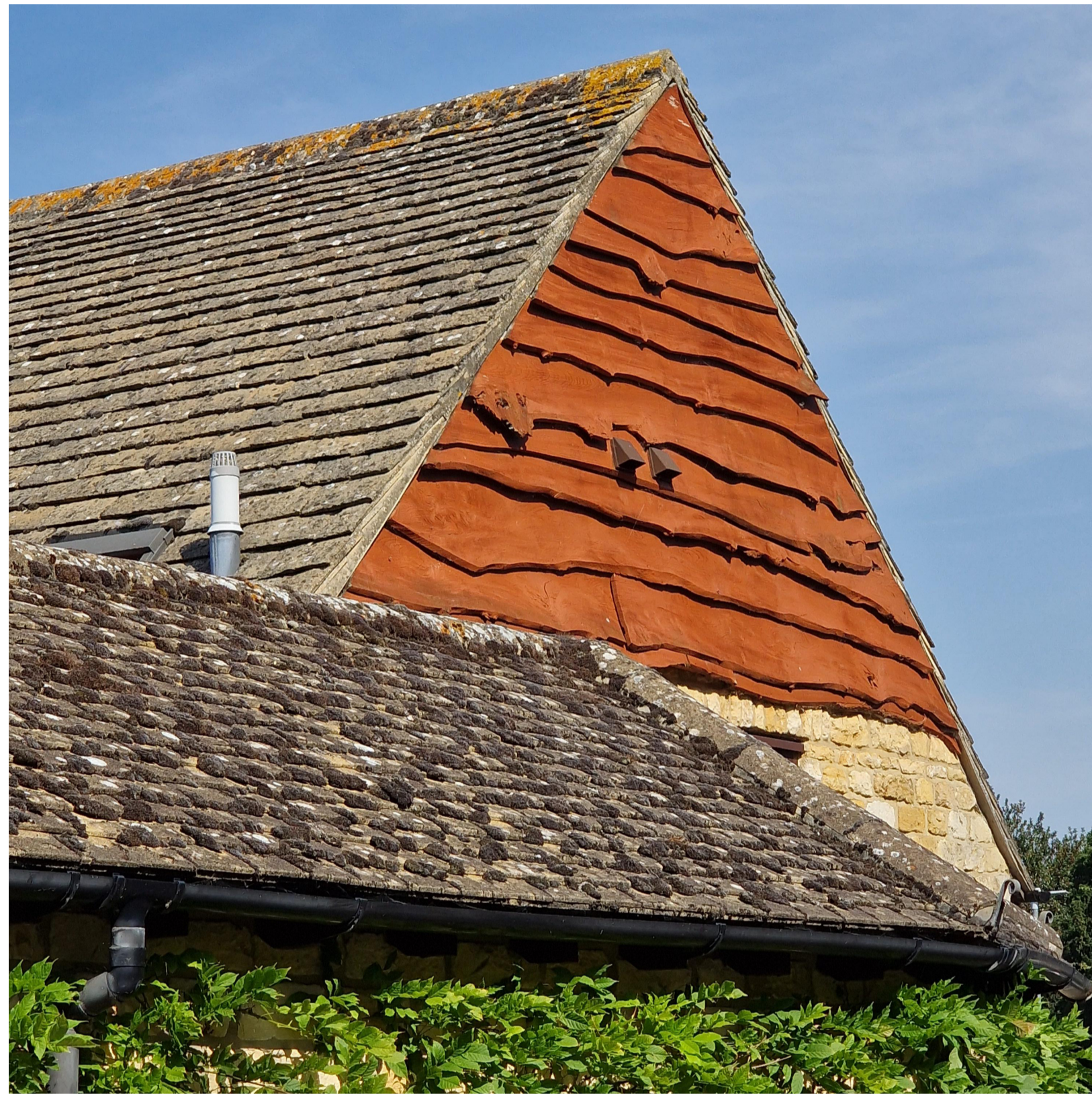
Example of waney edge boarding in Weston Subedge, within the Cotswold District Council conservation area
