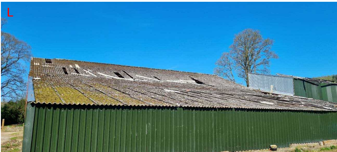
Damage to building.
