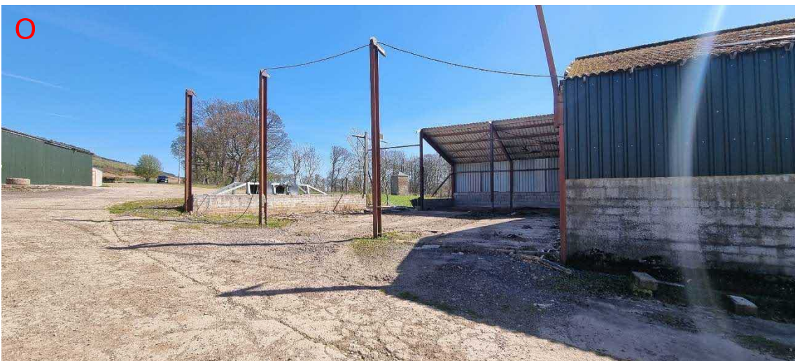
Roof taken off building by high winds
