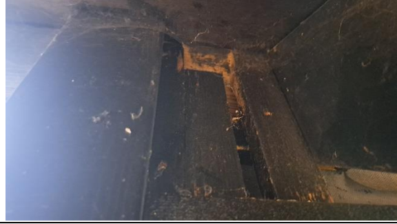
Photo 14 PRF at South east corner of roof - cavity behind timber boards. Bird droppings present
