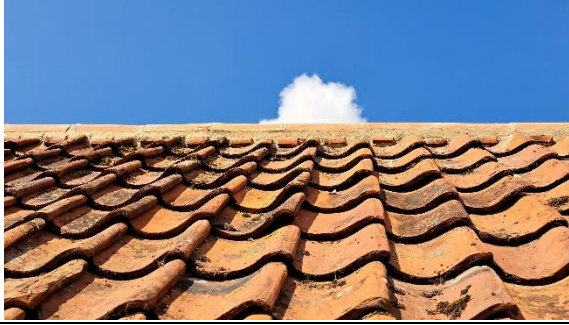
Photo 13 Pan tile roof - east elevation showing several raised tiles.
