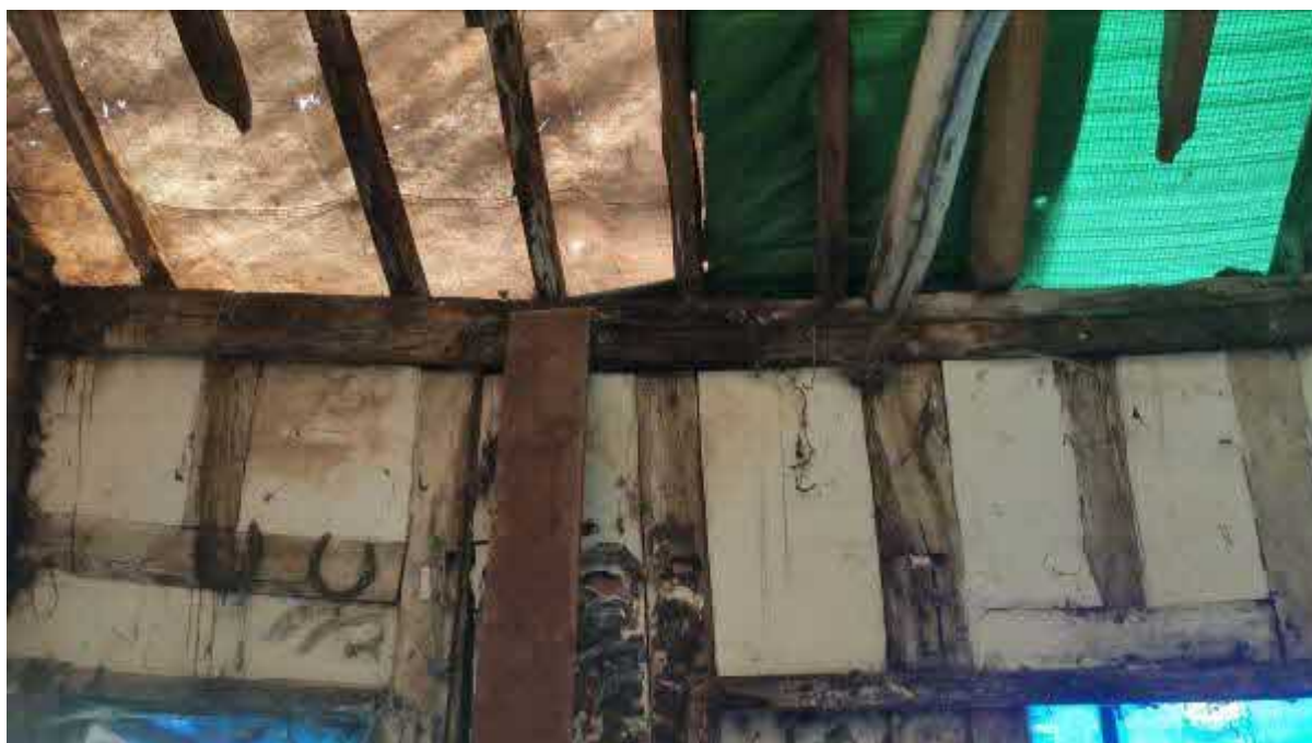
Photograph 07 – Condition of eaves plate/top rail, east facing elevation.
