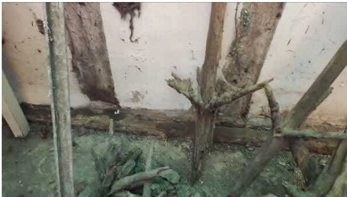
Photograph 09 – Previous cement repair to bottom timber plate, east facing elevation.
