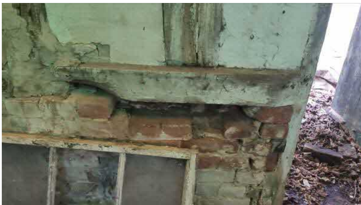
Photograph 18 – Missing bricks in plinth wall, west facing elevation.
