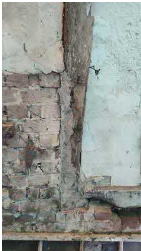
Photograph 16 – Previous cement repair to base of principal post, west facing elevation towards the south end.
