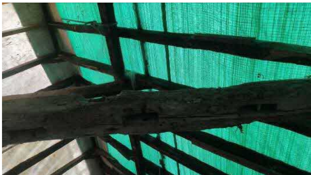
Photograph 04 – Split in tie beam nearest the south end.
