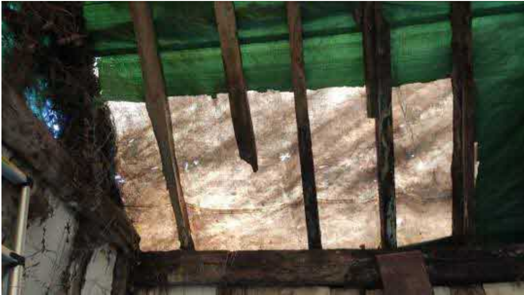
Photograph 01 – Snapped rafter on NE side.
