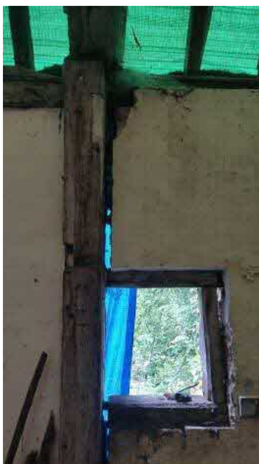
Photograph 08 – Principal post on east facing elevation at junction with later brick extension.
