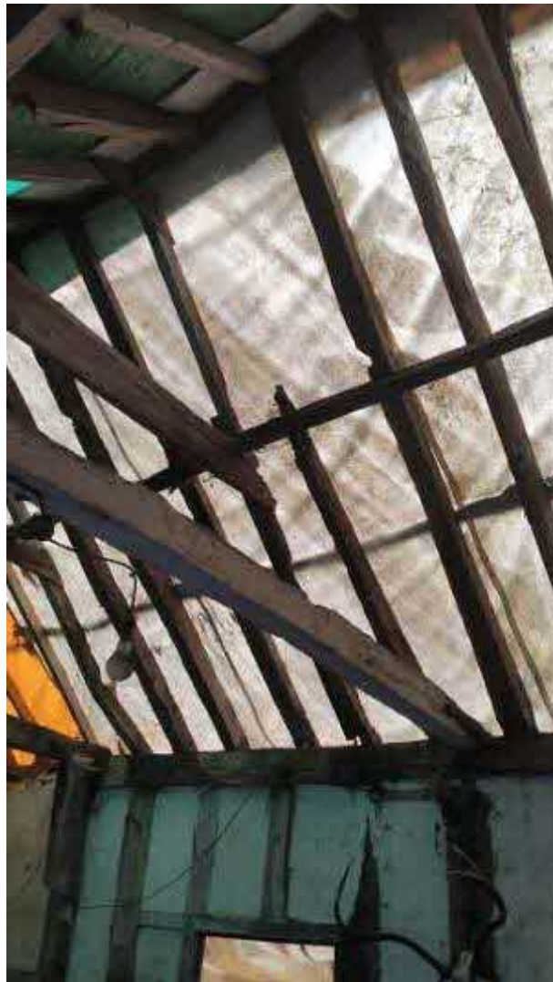
Photograph 02 – Damage to the west side of the roof.
