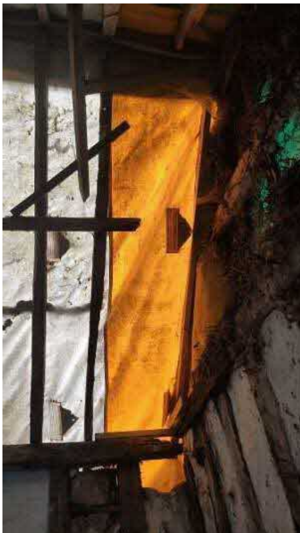
Photograph 03 – Missing rafter and purlin end. Also damage to joint between top rail and eaves plate, NW corner.
