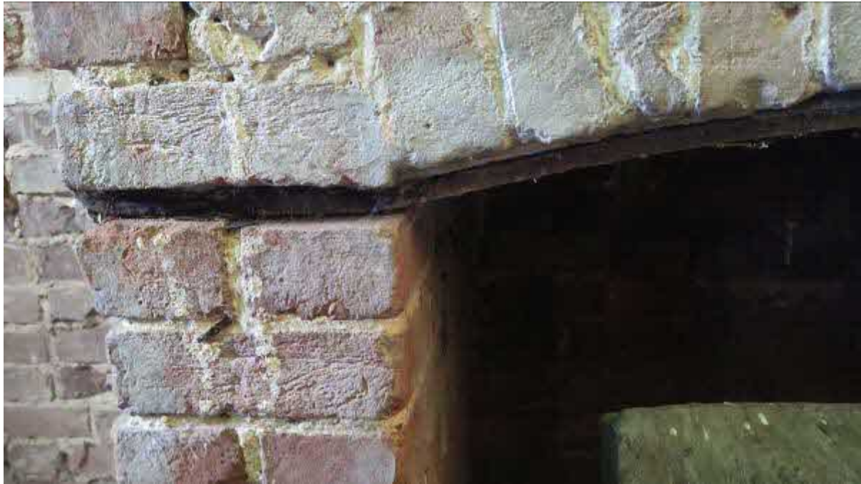
Photograph 13 – Rust jacking caused by the fireplace lintel.
