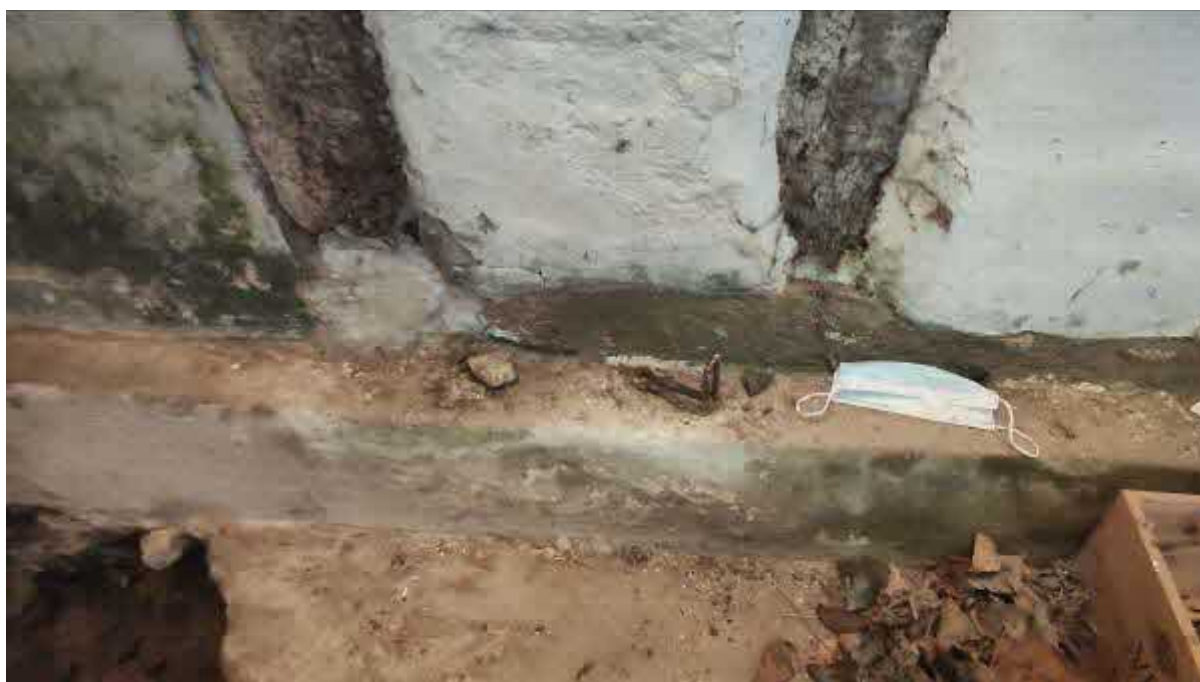
Photograph 06 – Concrete covered brick plinth wall and previous cement repair to bottom timber wall plate, north gable.
