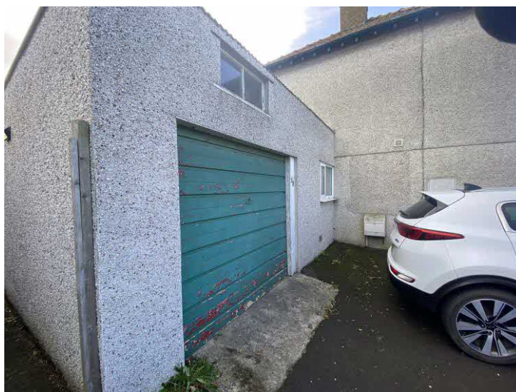
Figure 4. The north wall of the garage.
