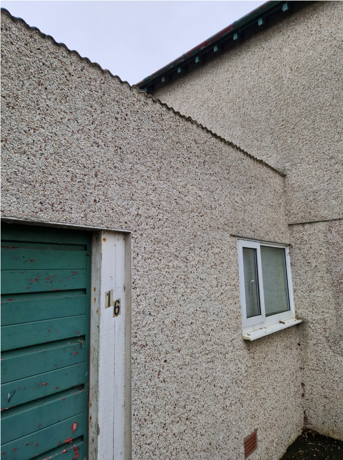
Front external northern wall and window where corrugated roof meets wall, clearly showing no gaps or crevices
