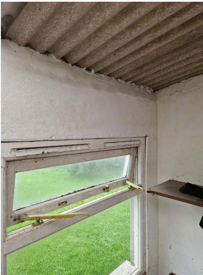
Internal rear wall and window showing no gaps or crevices
