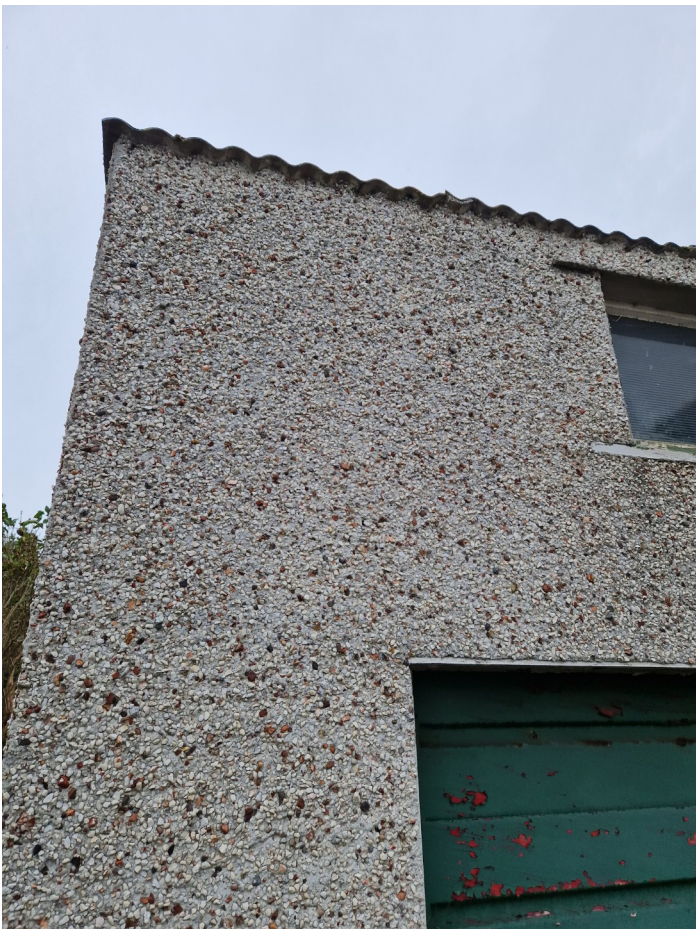
Front external northern wall where corrugated roof meets wall, clearly showing no gaps or crevices
