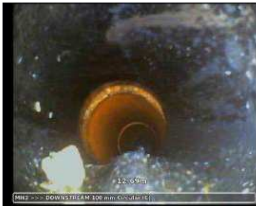
20221102-093611-snap0002.jpg, 00:01:01, 12.77 m Survey abandoned, Defect pipe
