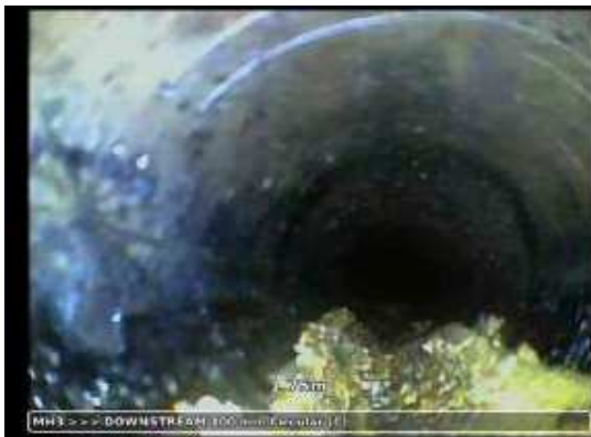
MH3X_eb4fd724-513f-48ce-a001-882928b98f4e_20221103_103640_938.jpg, 00:00:14, 1.75 m Settled deposits, other, 20% cross-sectional area loss, start
