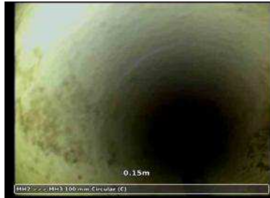
MH2X_d1e2fe50-4e31-4e78-b6c6-037906ac171f_20221103_102714_032.jpg, 00:00:05, 0.15 m Crack, circumferential from 9 o'clock to 3 o'clock
