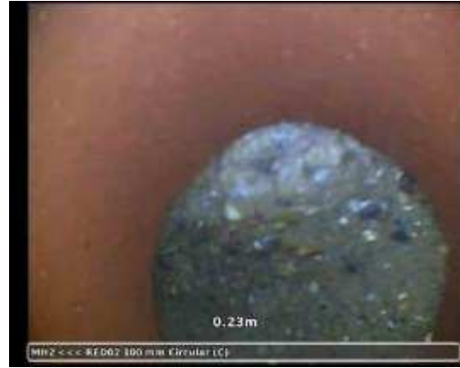
20221102-091350-snap0001.jpg, 00:00:09, 0.23 m Finish node, major connection without manhole, reference: RED02
