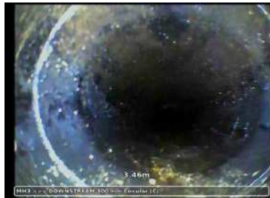
MH3X_ec6b3537-449e-418a-849f-c58954c1dc25_20221103_103658_450.jpg, 00:00:19, 3.46 m Settled deposits, other, 20% cross-sectional area loss, finish
