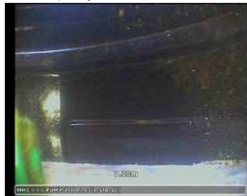
20221102-083441-snap0002.jpg, 00:00:37, 7.30 m Finish node, other special chamber, reference: PUMP, PUMP STATION
