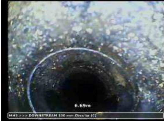
MH3X_e584b10d-6e36-4463-a30e-b638d0b97122_20221103_103825_879.jpg, 00:00:32, 6.69 m Deformed drain or sewer, 20%, start
