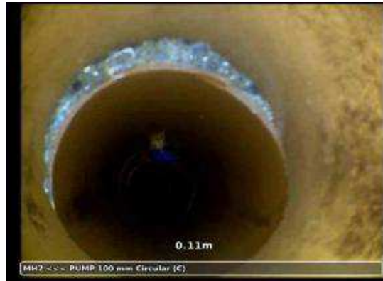
PUMPX_3e4c5767-e416-4097-99d1-cd8b95deb938_20221103_101803_237.jpg, 00:00:07, 0.15 m Joint displaced, large
