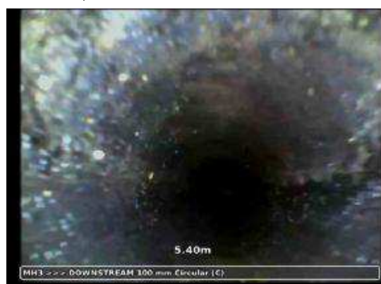
MH3X_bbb910b0-a049-4d7a-94b2-b81635bf3c1a_20221103_103755_390.jpg, 00:00:28, 5.32 m Deformed drain or sewer, 15%, start
