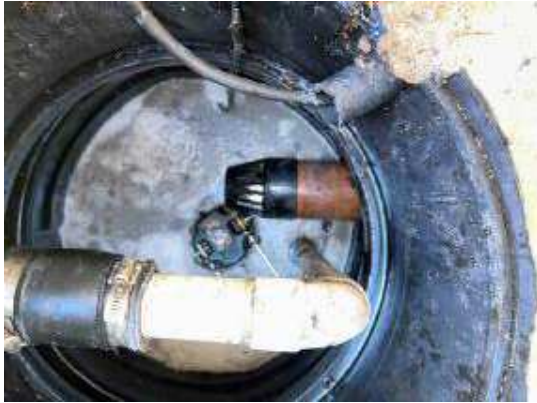
Recommend to remove Birdsnest off MH1 outlet in pump station due to blocking system
