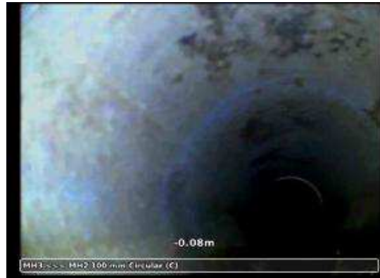
MH2X_263d938a-33ac-4c5d-af43-acc89c52318e_20221103_103027_801.jpg, 00:00:05, 0.08 m Crack, circumferential from 12 o'clock to 12 o'clock
