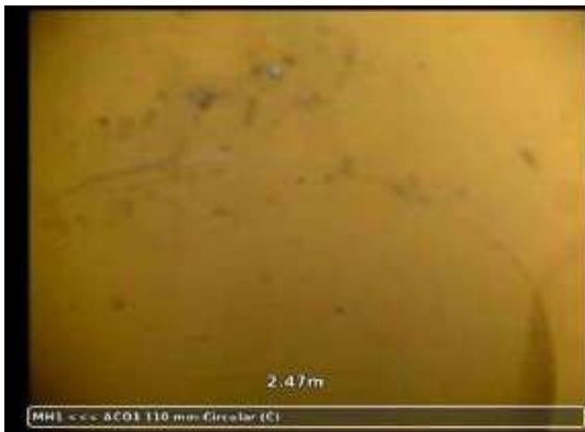
ACO1X_0a4b3754-92b0-40fb-acc1-091df3d48932_20221103_ 101148_421.jpg, 00:00:14, 2.47 m Line deviates down
