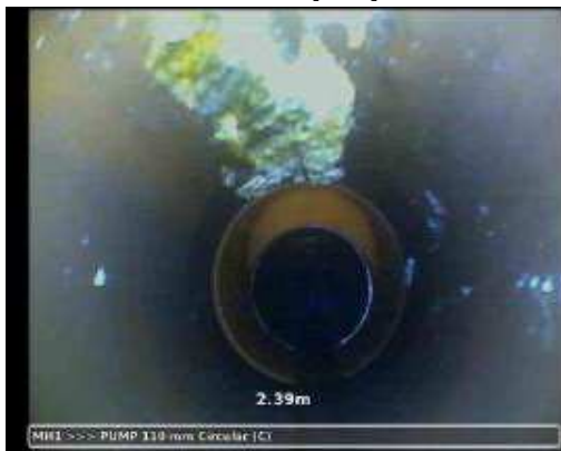
20221102-083441-snap0001.jpg, 00:00:17, 2.39 m Junction at 12 o'clock, diameter: 110mm, CWG1
