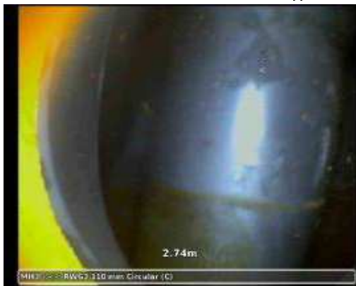
20221102-092841-snap0002.jpg, 00:00:18, 2,74 m Finish node, gully, reference: RWG3
