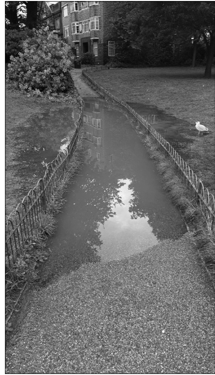
Existing drainage issue
