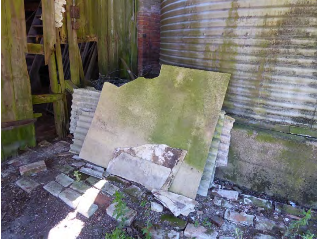
Plate 11: Asbestos sheets adjacent to silo
