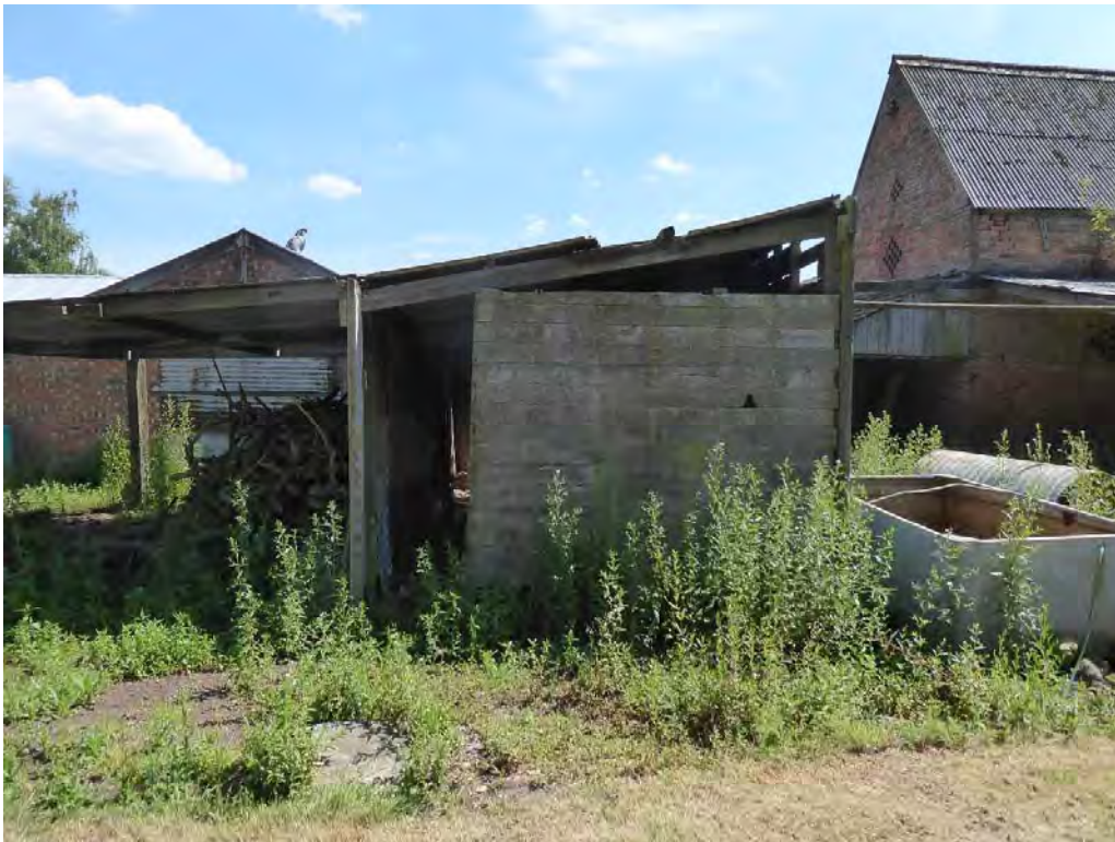
Plate 8: The rear lean-tos and outbuildings
