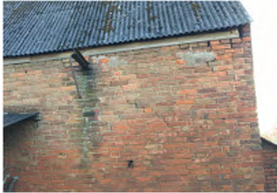
Crack at rear external corner
