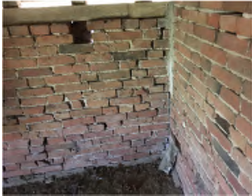
Wall crack at corner of part mezzanine
