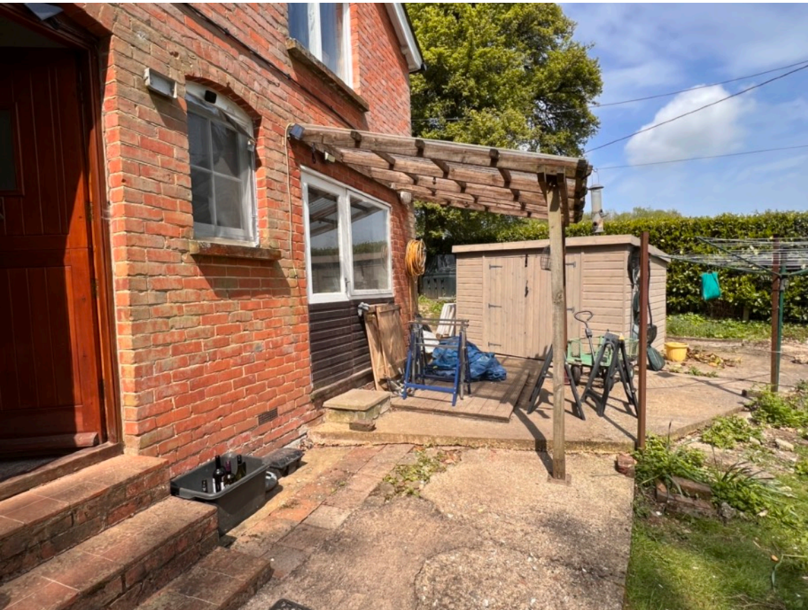
Fig. 5. Concrete hardstanding to rear elevation
