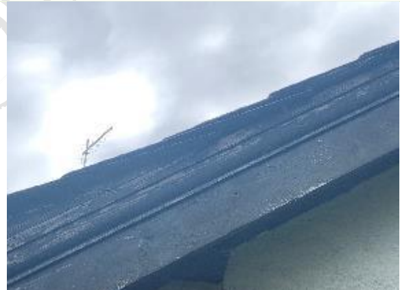
Gaps under the slate verge – potential bat access
