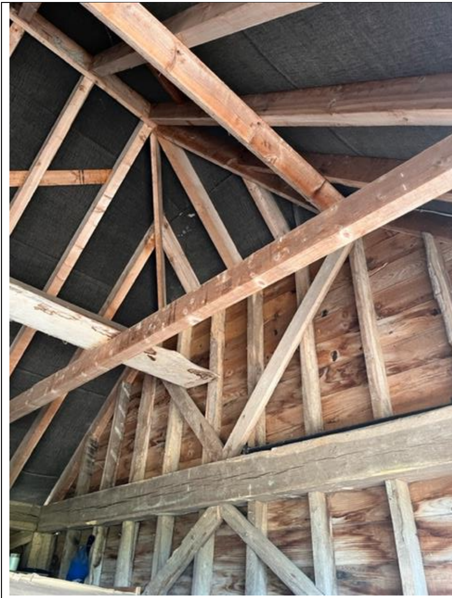
PHOTOGRAPH 20: Close up of the underside of the Garage roof showing the roof trusses and the black under felt.
