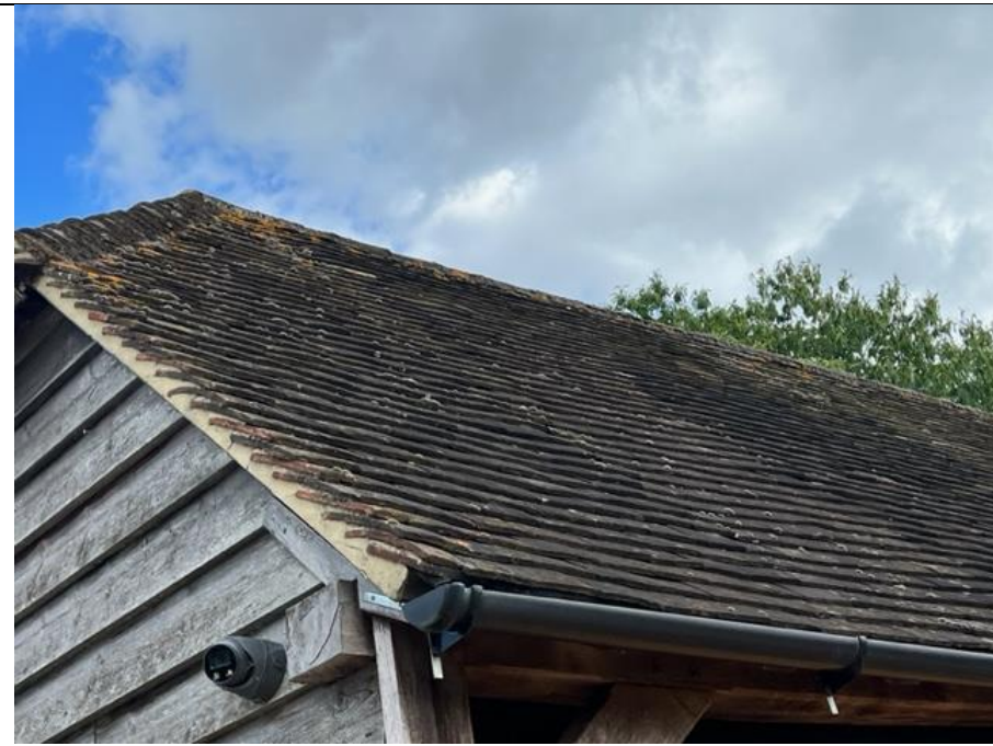
PHOTOGRAPH 16: The east facing gable of the Garage showing the weatherboarding and the sealing of the tiles.
