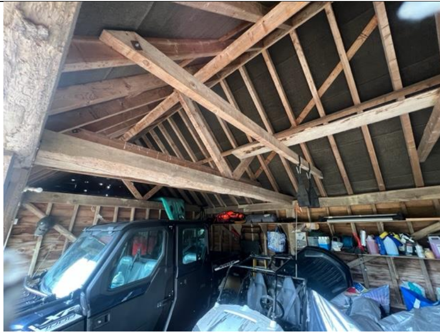
PHOTOGRAPH 19: The underside of the Garage roof showing the traditional black under felt.
