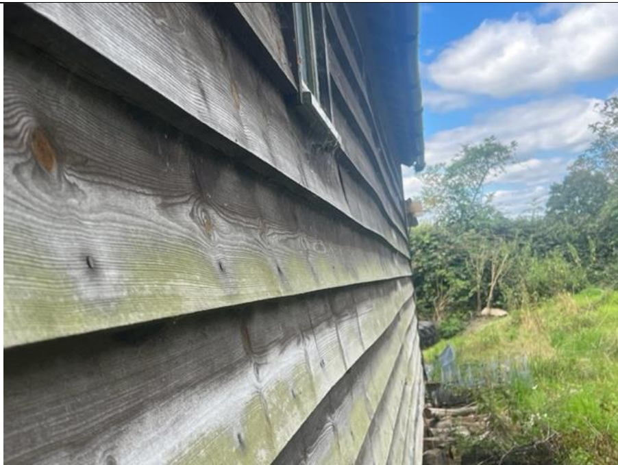
PHOTOGRAPH 12: A close up photo of the weather boarding of the Annex and Gym.
