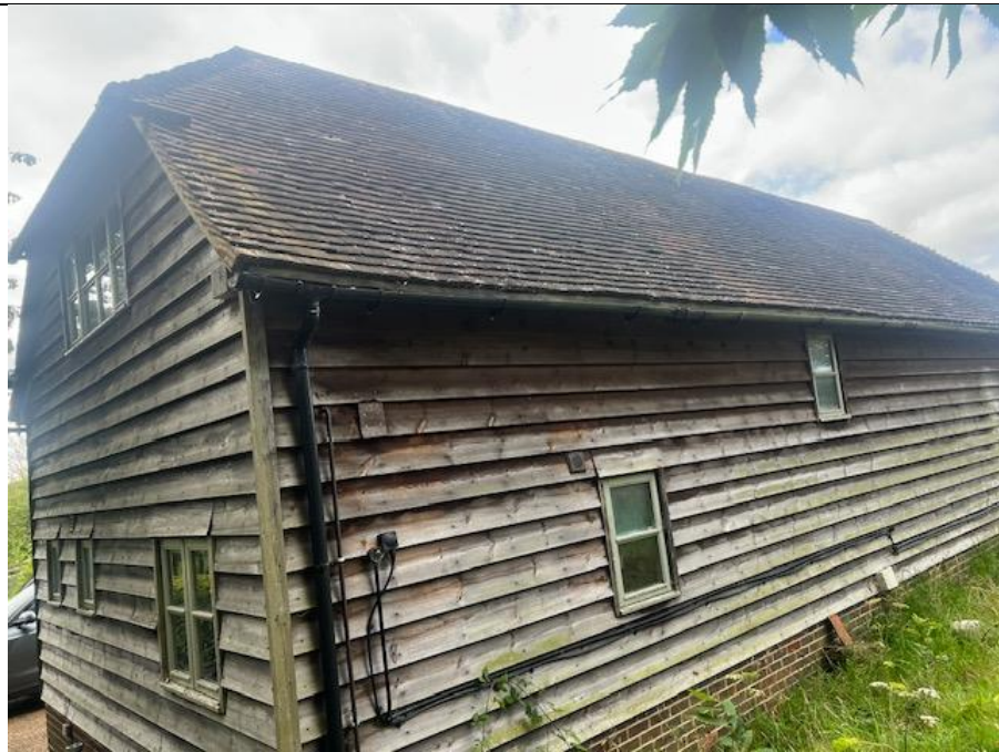
PHOTOGRAPH 4: View of the east and south elevation of the Gym and Annex.
