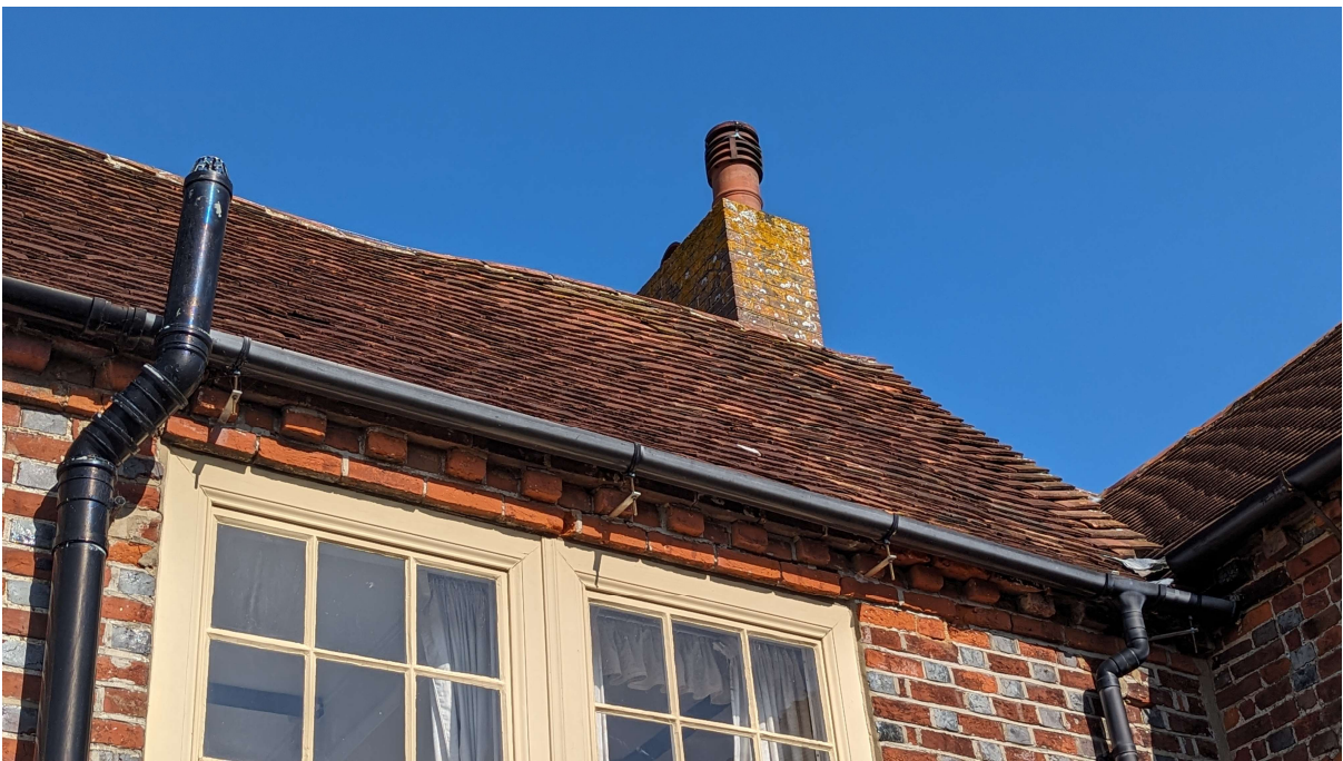
Photo 3 – View of the gappy roof tiles to the rear.
