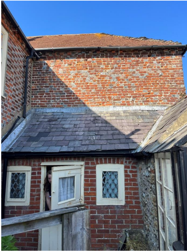
3. South elevation of existing single storey extension (neighbouring Crab & Lobster pub in the background).
