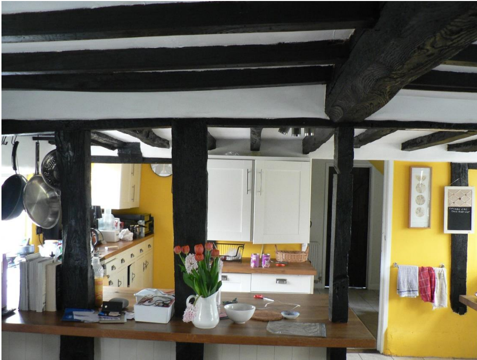
Figure 10. View showing the existing black treatment to the ground floor historic timber frame members
