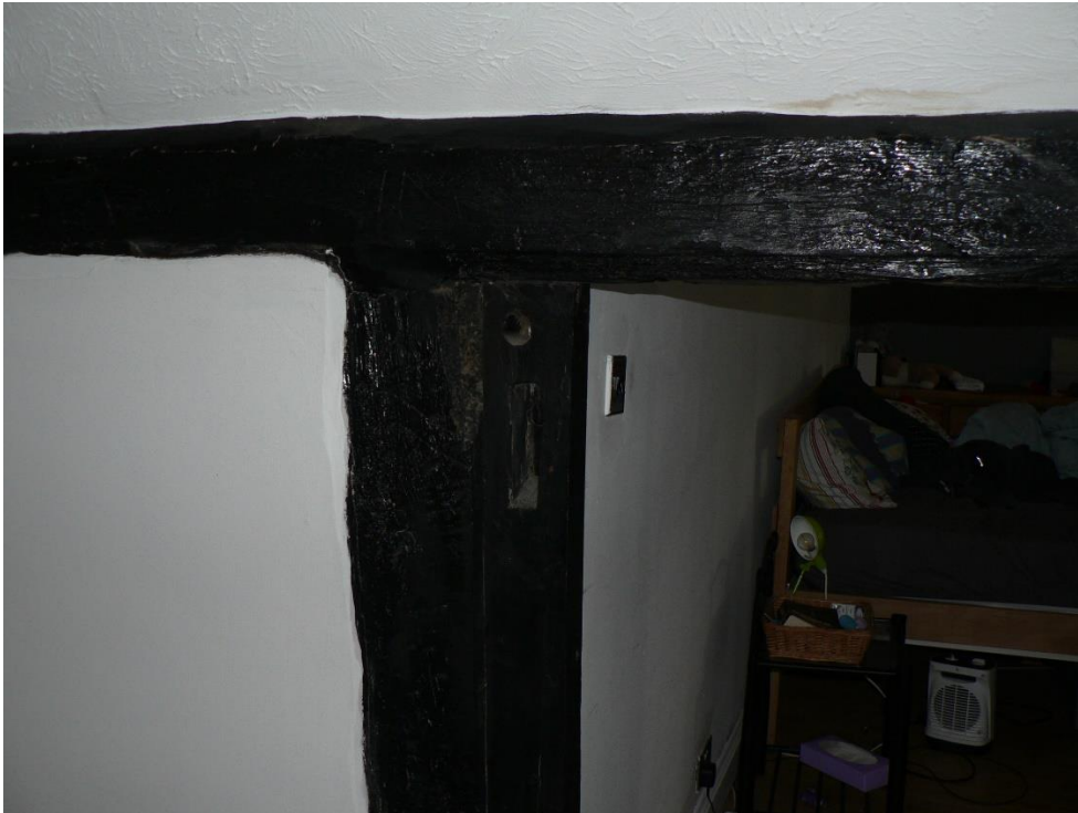
Figure 6. View showing the existing black treatment to the first floor historic timber frame members
