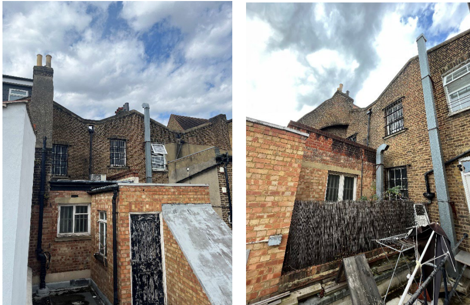
Simple and outdated exterior elements – 212 High Street
