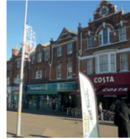
176- 186 High Street Year: 1898 Materials: Red Stock brick Windows Sash Flemish and Queen Anne-style influences.
