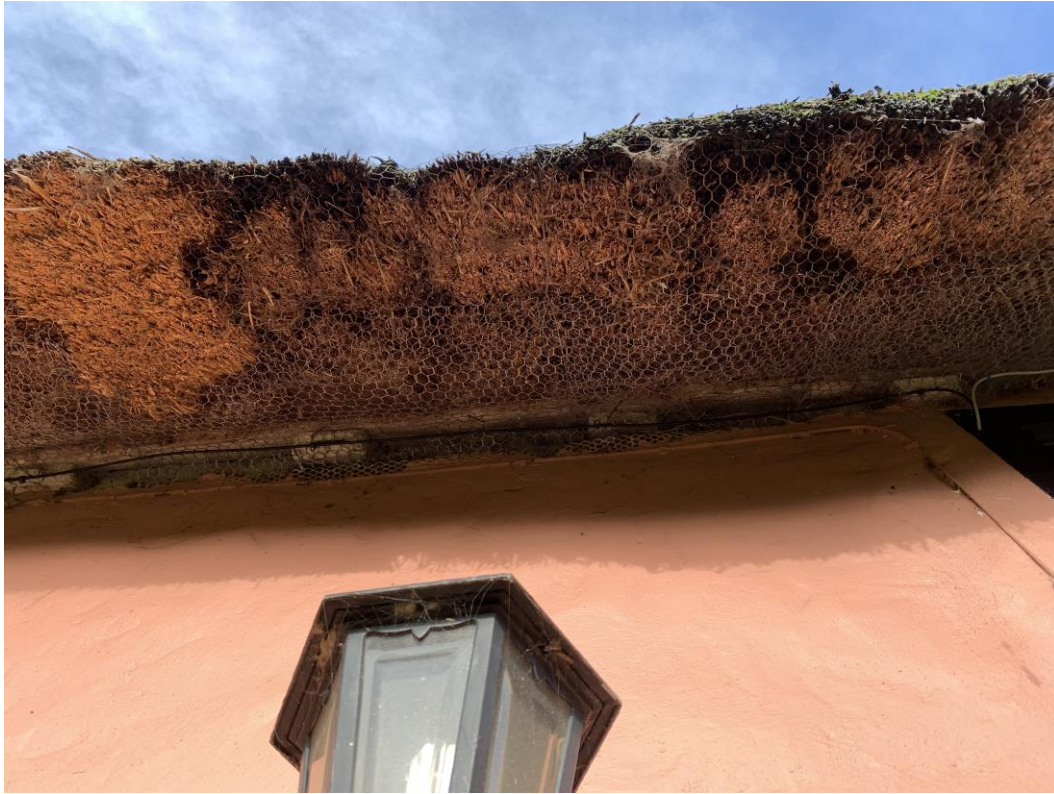
Plate 3: Eaves above proposed new porch – fully wired onto the rendered wall (Photo: O. Robson, 30/10/23)
