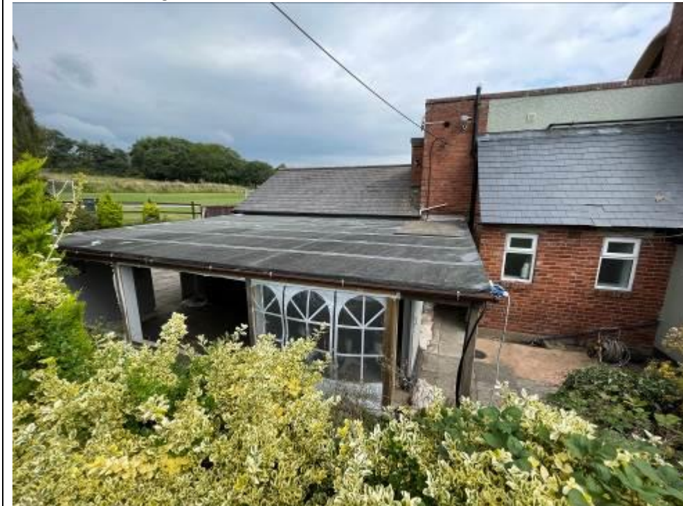
View from the beer garden on to the top of the existing flat roof extension
