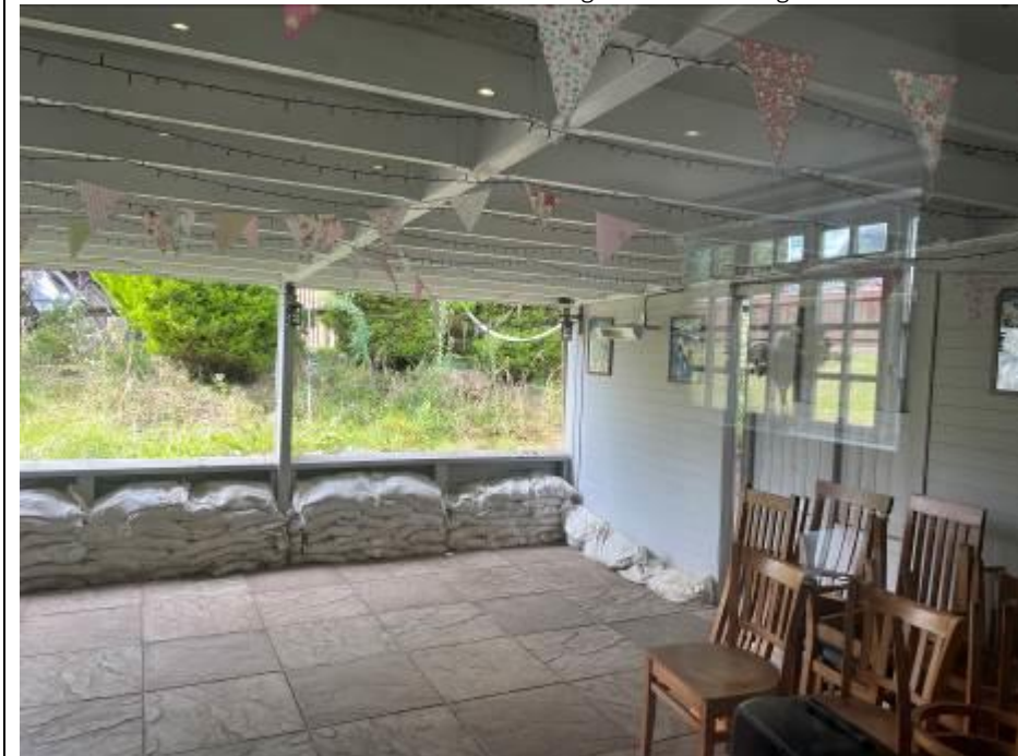
Photo taken inside the flat roof extension looking out on to beer garden and to the right sliding barn door access to patio area – shows sand bags due to surface water run off
