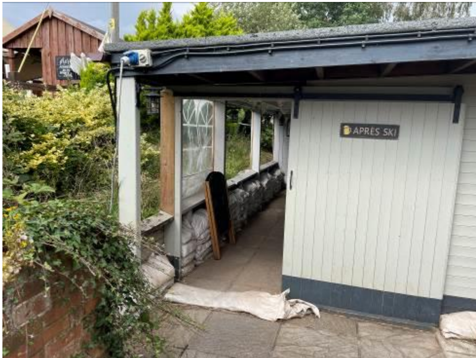
View from the road side elevation to the side of the existing flat roof extension
