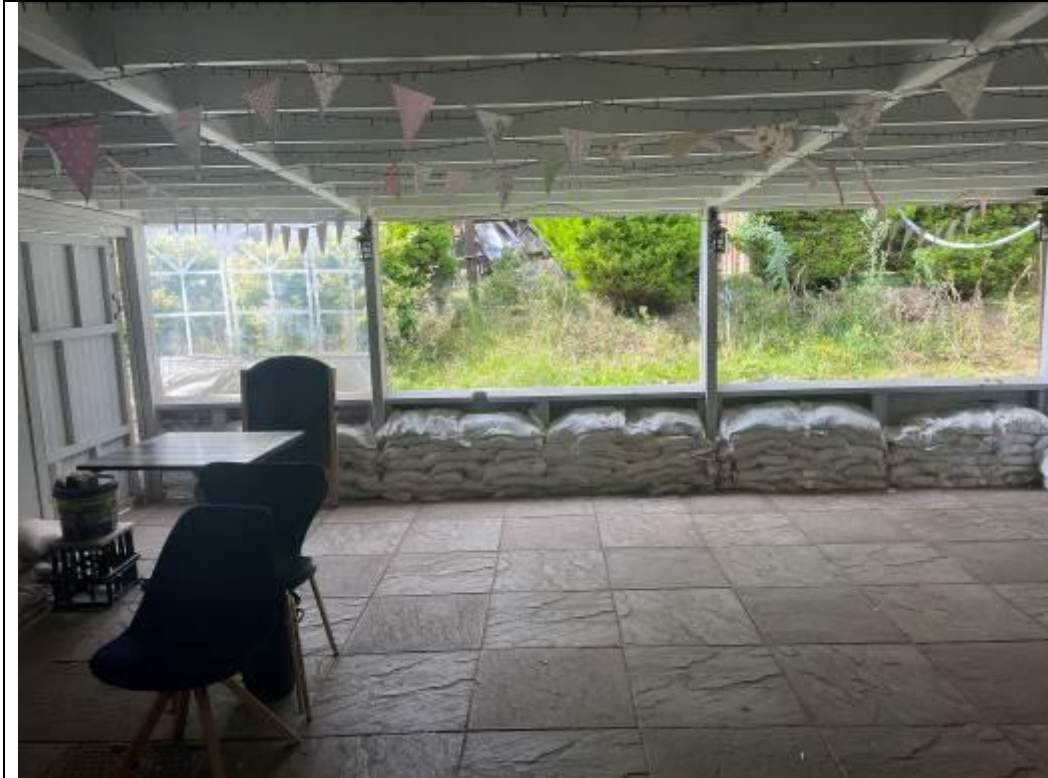
Photo taken inside the flat roof extension looking out on to beer garden – shows sand bags due to surface water run off
