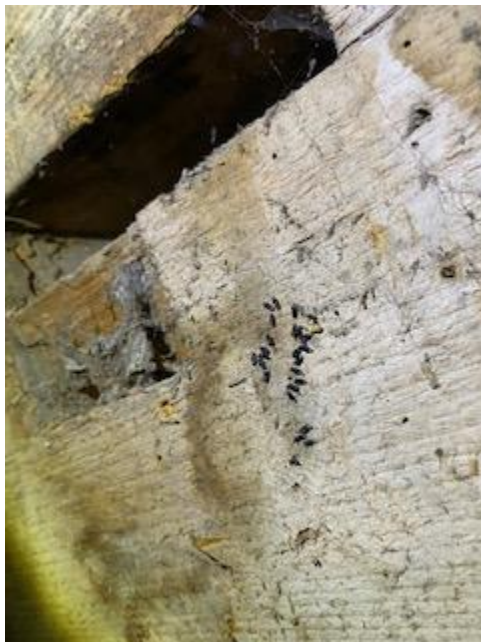
Photograph 3 – old bat droppings found attached to timber beam in loft space of building.
