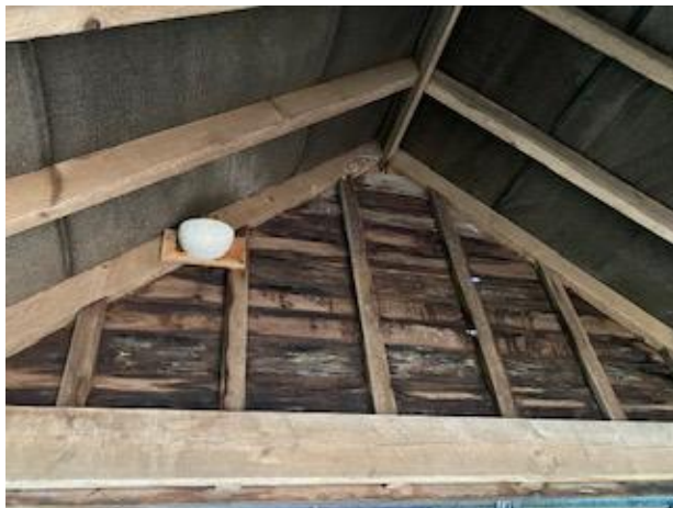
Photograph 10 – internal of car port with swallow cup and part of a natural swallow nest at the pitch of the roof.
