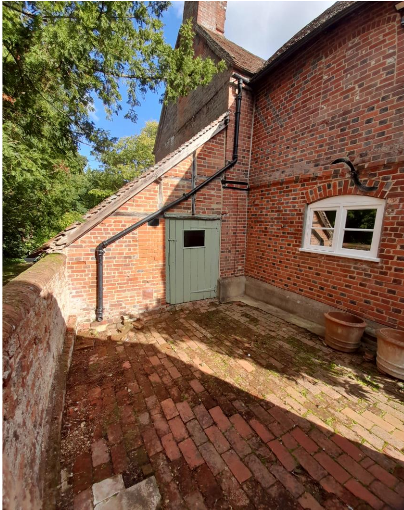
Fig. 8: View, looking north-east, of the north-west, side elevation of Church Farm House, with the lean-to addition and brick-paved yard.
