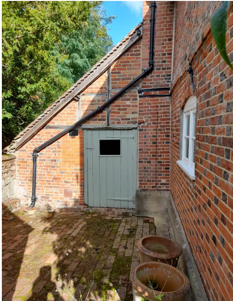
Fig. 16: View, looking north-east, if the south-west elevation of the lean-to on the north-western side of the house, and the proposed location of the extension.
