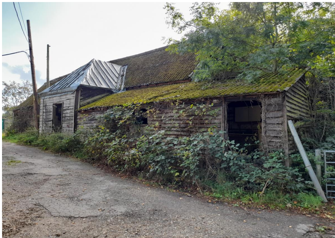
Fig. 18: View, looking south, of the front elevation of the Grade II-listed barn at Church Farm.
