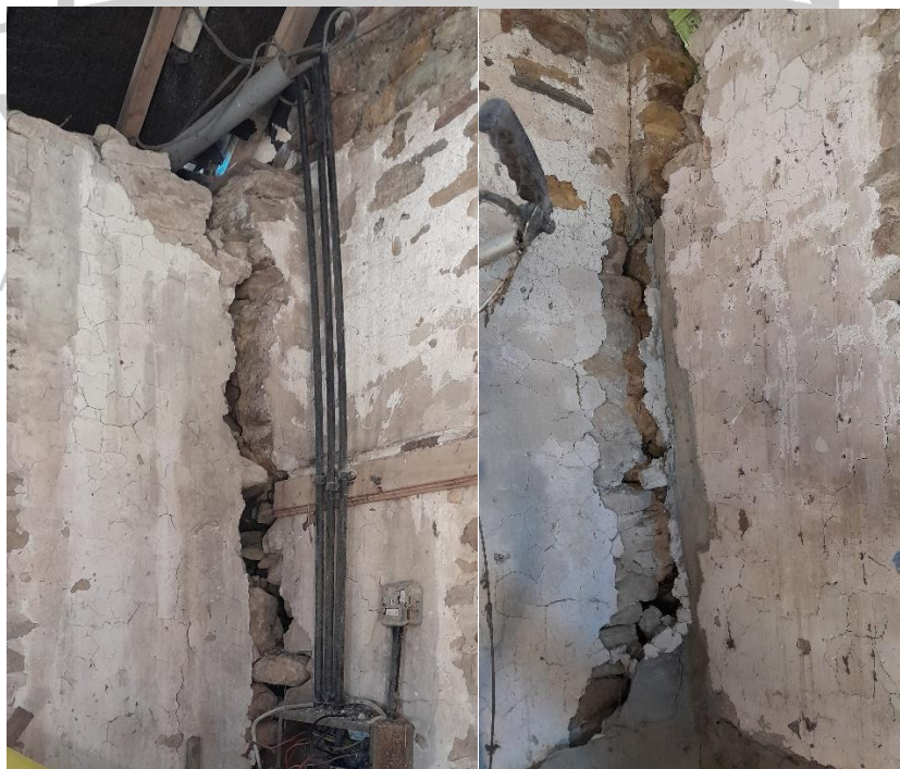
Photo 7: Cracking at the eastern corner Photo 8: Cracking at the southern corner
