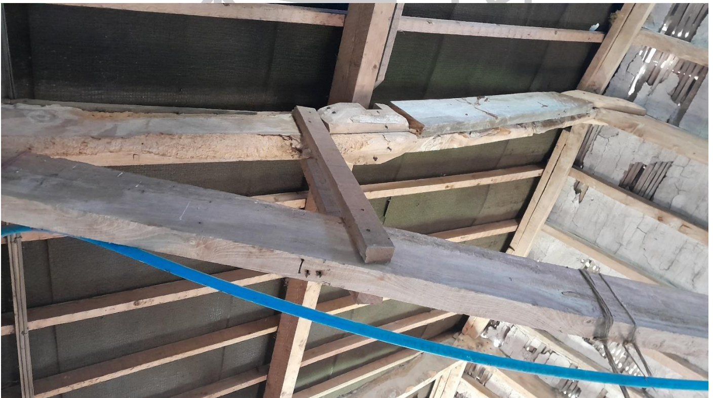
Photo 3: Timber decay on truss rafters and previous repairs
