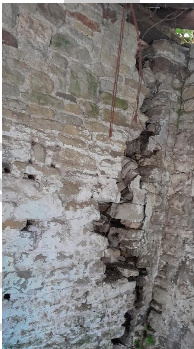
Photo 9: Cracking at the east corner of the timber lean-to
