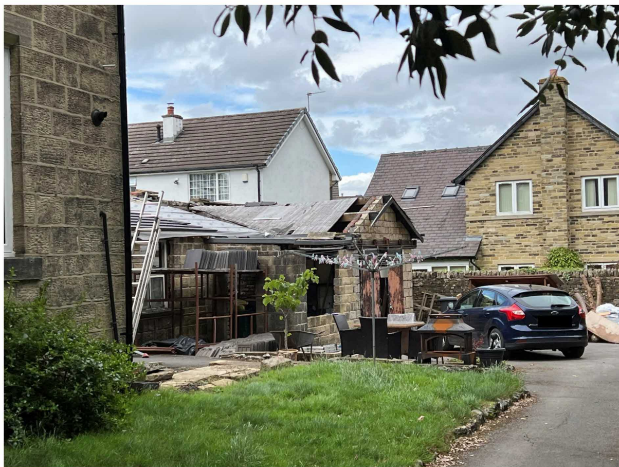
The existing outbuilding in its current state of dilapidation.
